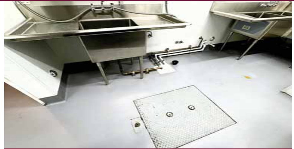
In-Ground Grease Interceptor
