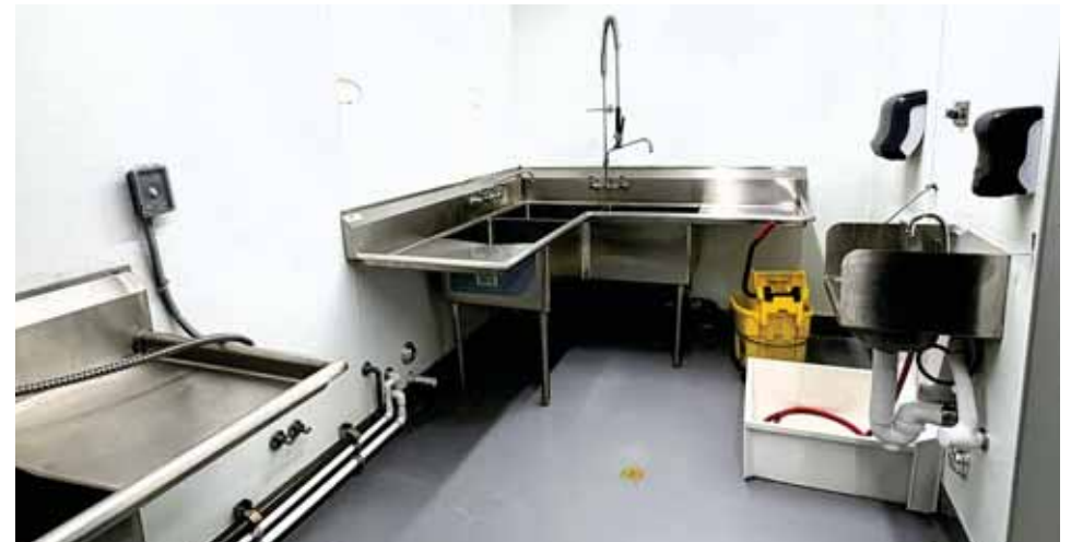
Stainless Steel Compartment Sinks and Mop Sink
