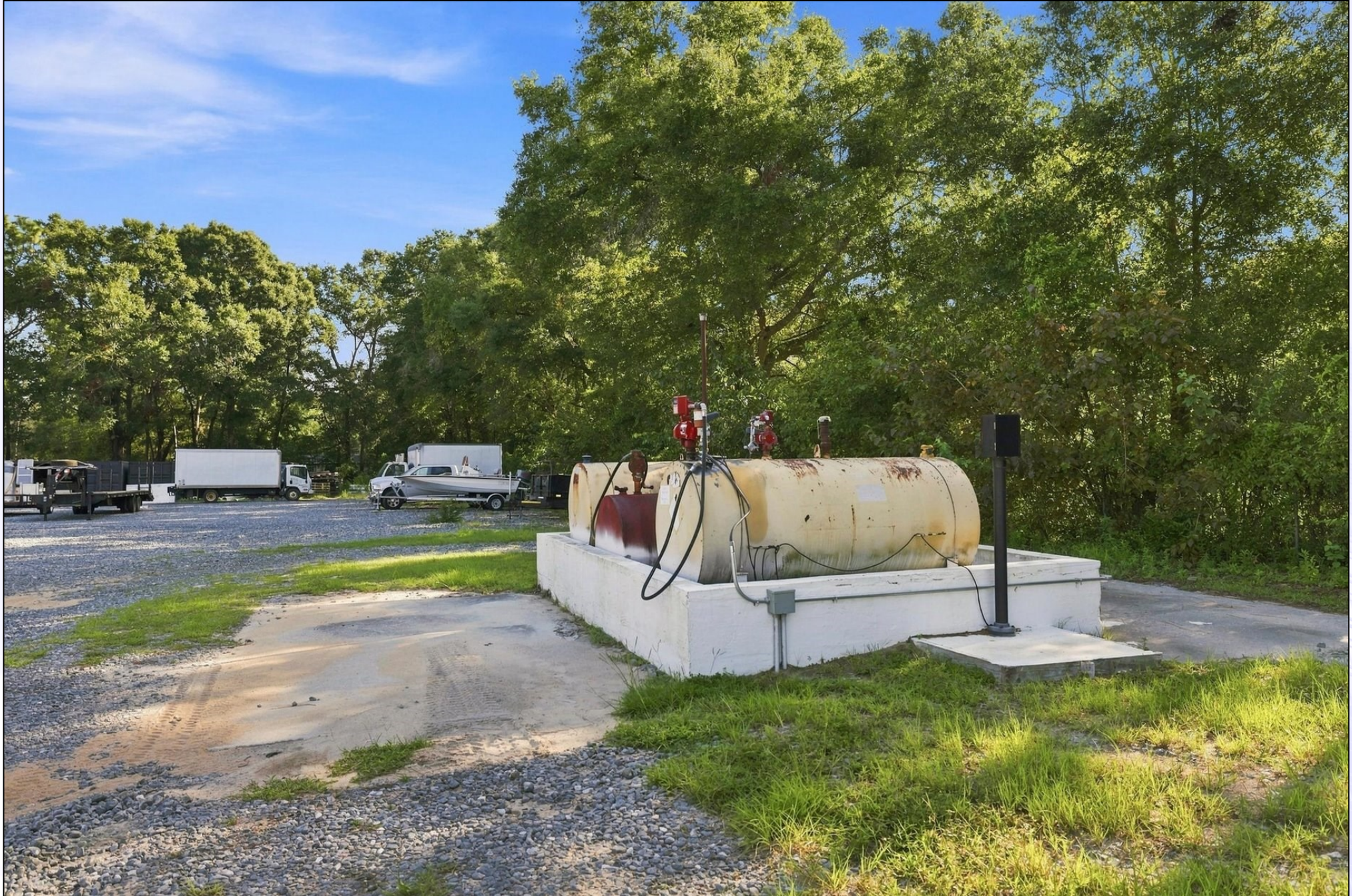
Fuel Island with Containment
