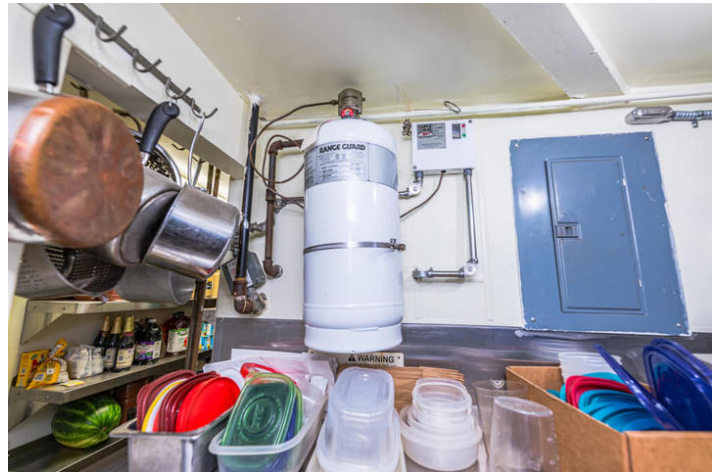
Protect your kitchen with this fire suppression system.
