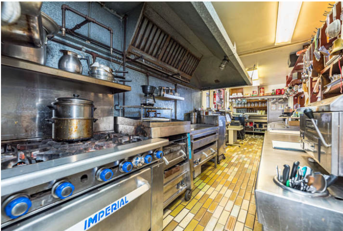
Fully equipped hot line and hood!
