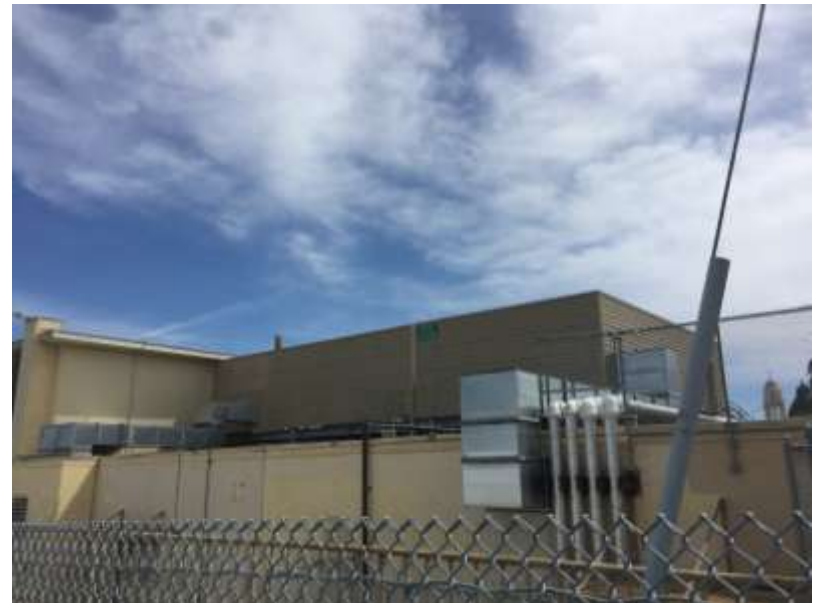
Photo 8: View of generator diesel "belly tank" located on top of the adjacent AT&T building
