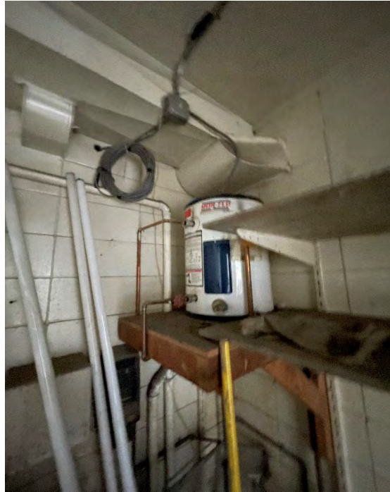
9. Representative view of hot water heaters at the site.
