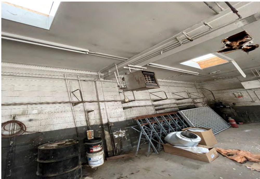
12. Representative view of ceiling mounted heating units, light bulbs/ballast and air compressor observed at the site.
