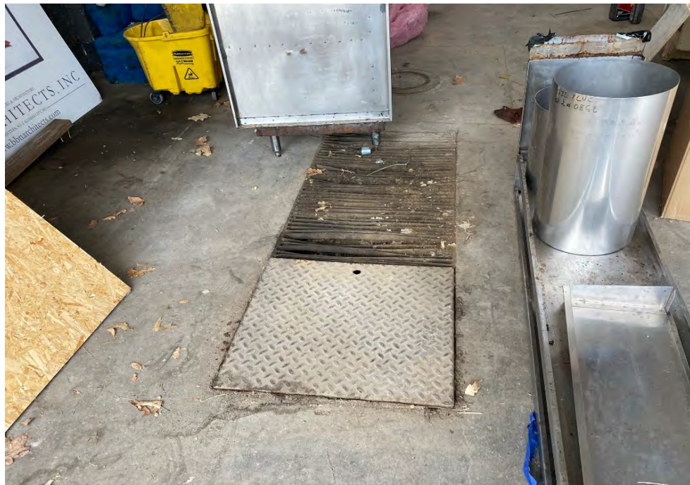
8. View of oil/water separator in the north bay of the building.
