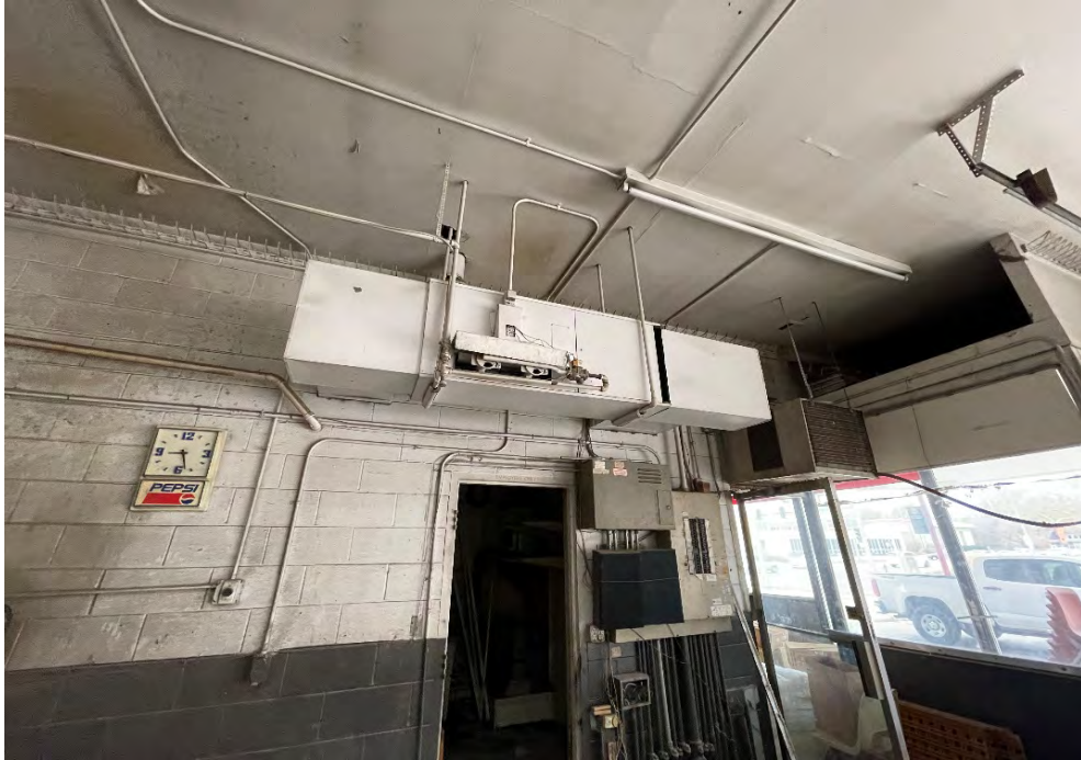
7. Representative view of retail HVAC within the building.
