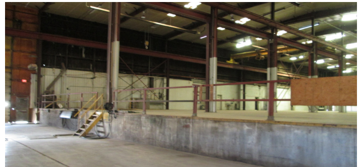
INTERIOR DOCK AREA SERVES 5 TON AND 10 TON CRANE BAYS
