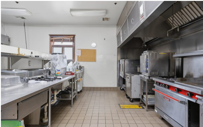
Commercial kitchen with hood, cooking line, ovens and prep areas.
