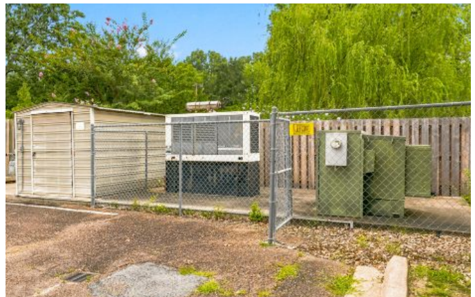
Ample power on site, with a standby generator installed alongside the building transformer in the screened service court.
