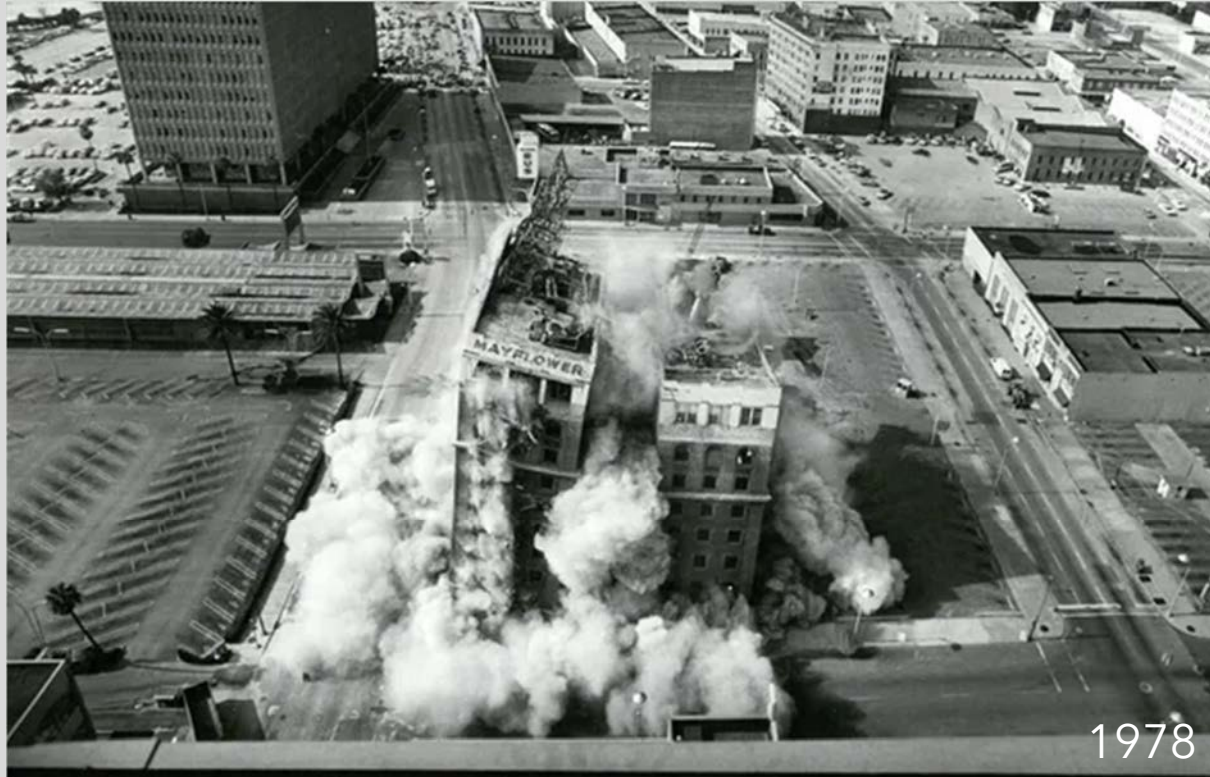
The 200 room, Mayflower Hotel at 301 W Bay is demolished after sitting vacant for seven years and is the first building implosion in downtown Jacksonville.
