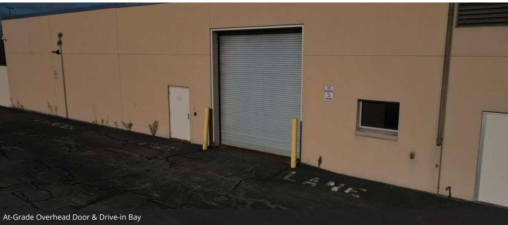
At-Grade Overhead Door
