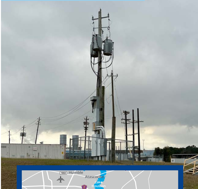
Heavy Power Connections for fabrication
