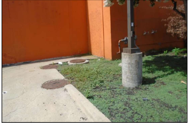
8 – View of the grease trap located behind Chacos.
