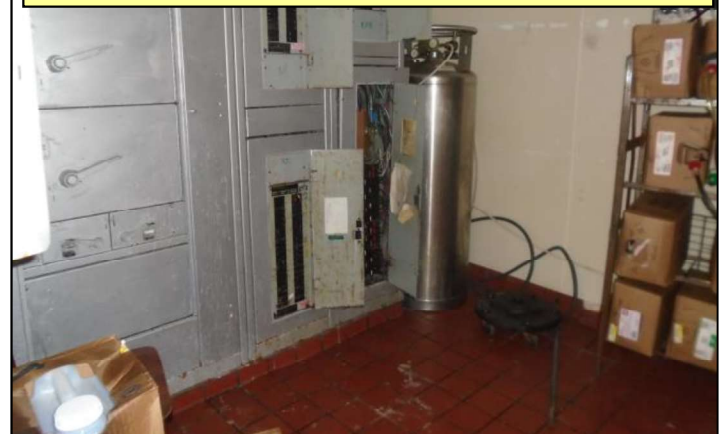
30 – View of the electrical panel located in the storage room.
