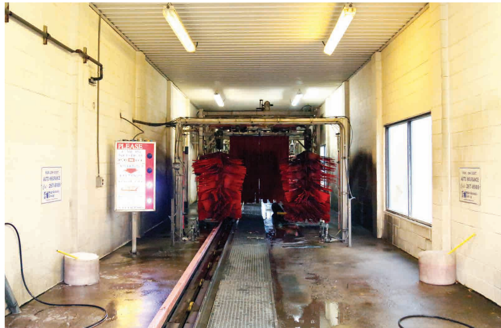
Automatic Wash (2) Tunnel
