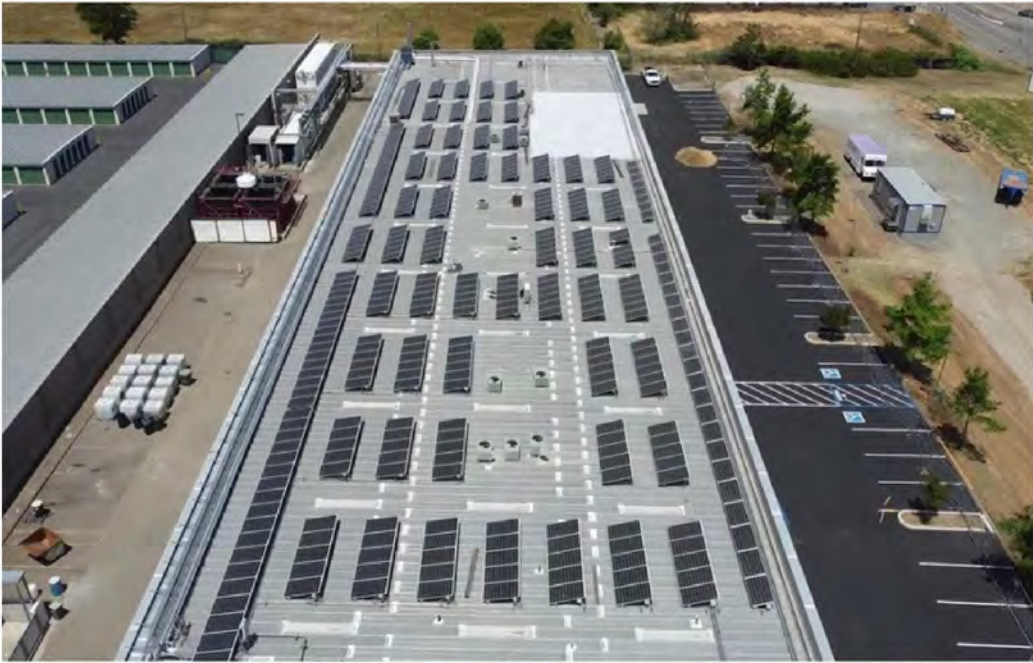
Roof Mounted Photovoltaic System
