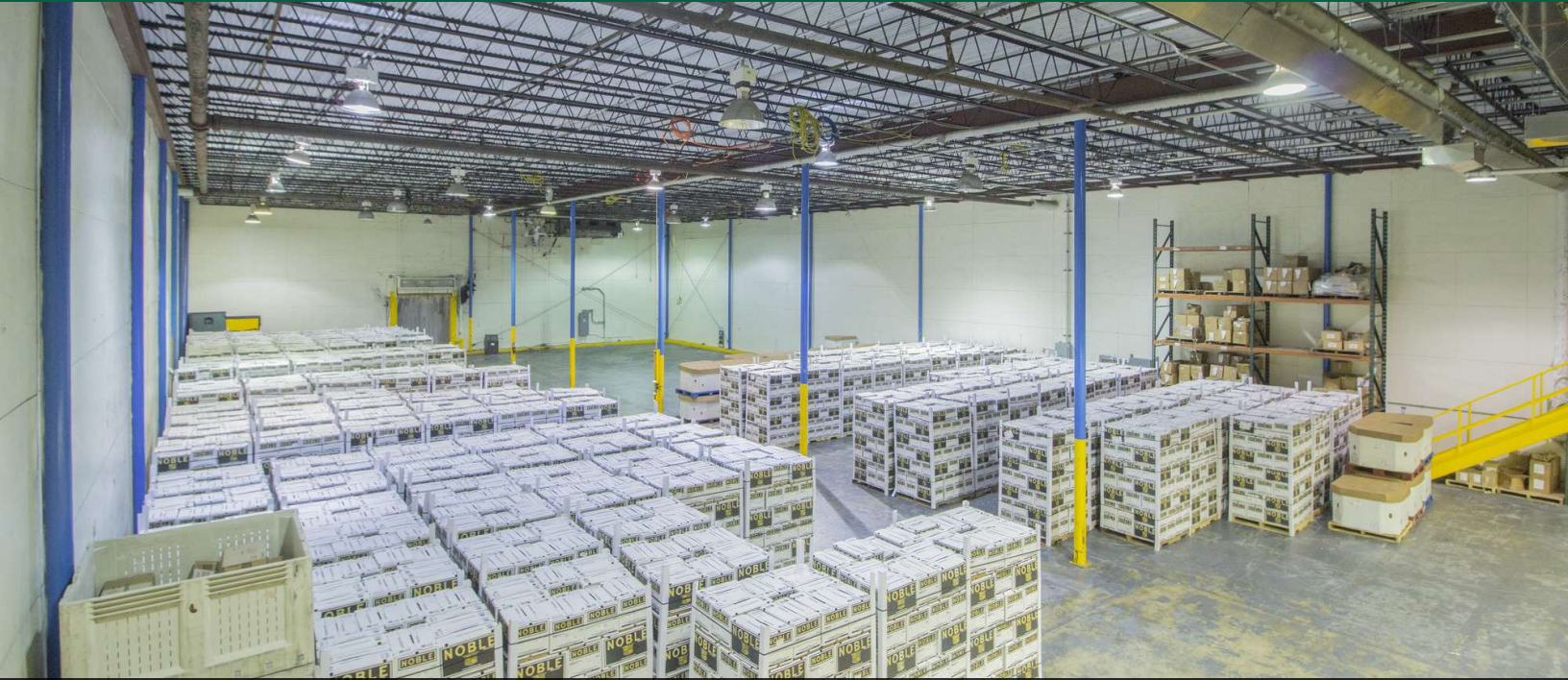
Cold Storage - Room A
