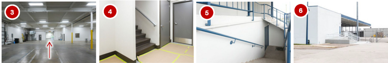
3. Fire Door Separating Climate Controlled and Open Air Warehouse Spaces
