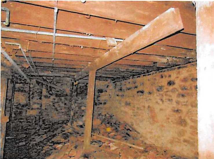
18. Another support post and column location that are rolling and tipping due to the extensive deterioration and rot problems.
