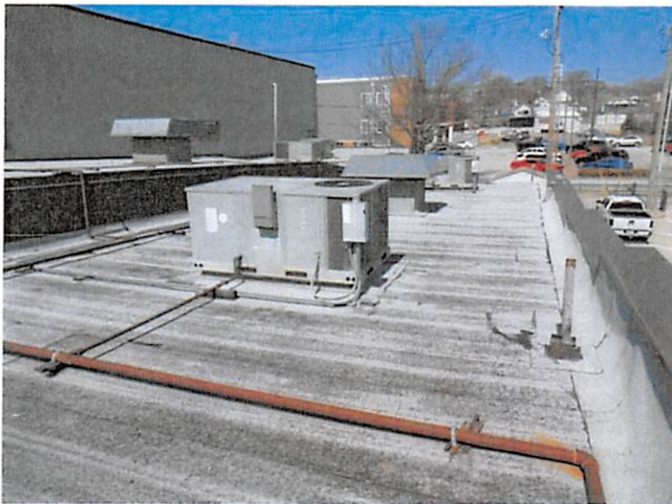
22. Looking north on the roof of the east half of the building.
