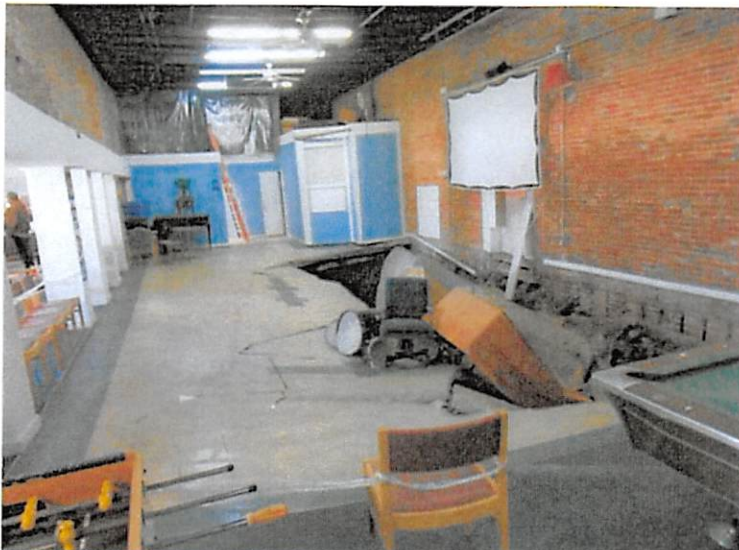
6. Looking south at the collapsed floor in the western half of the building.
