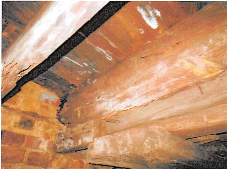
14. Extensive deterioration, rot, and termite damage in the joists closer to the south end of the east side.
