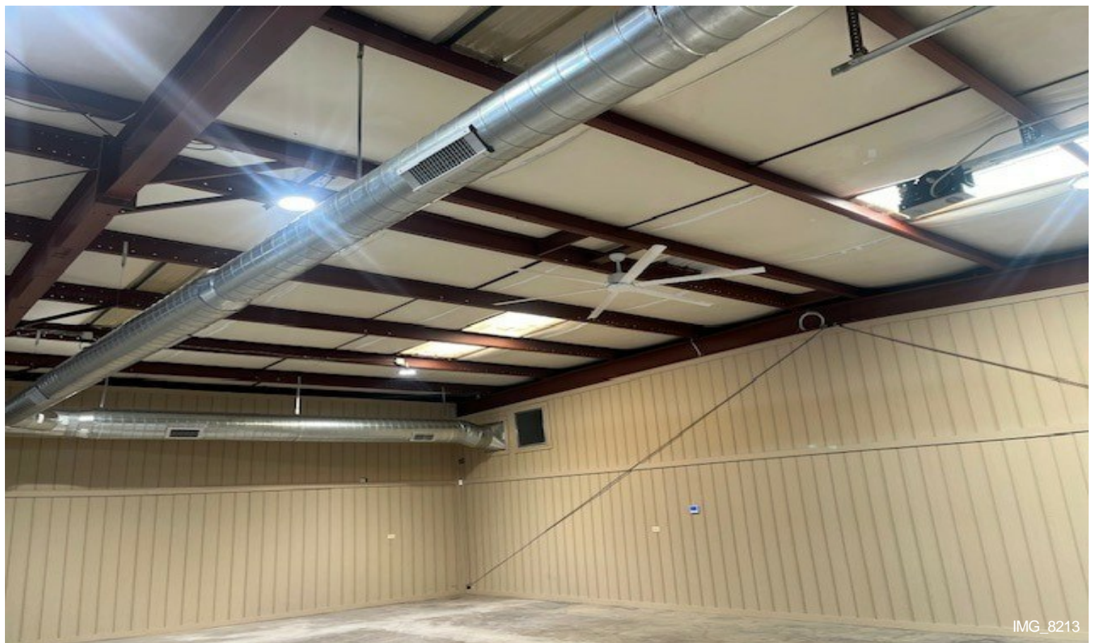
Warehouse includes new lighting, HVAC ducts and large fan
