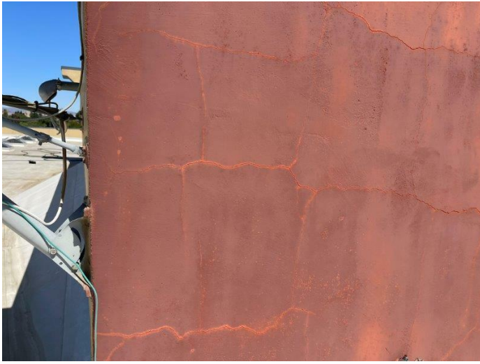
55. Rooftop, mezzanine penthouse: damaged stucco.
