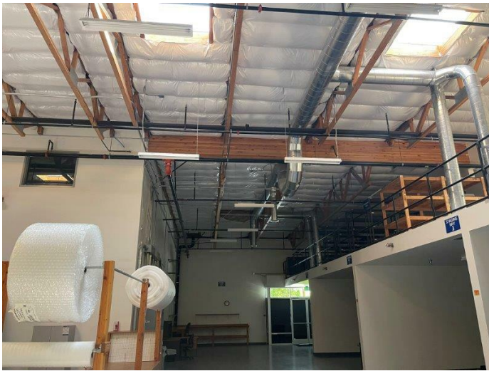
19. Roof framing appears to be glulam joists and wood beams covered with oriented strand board.
