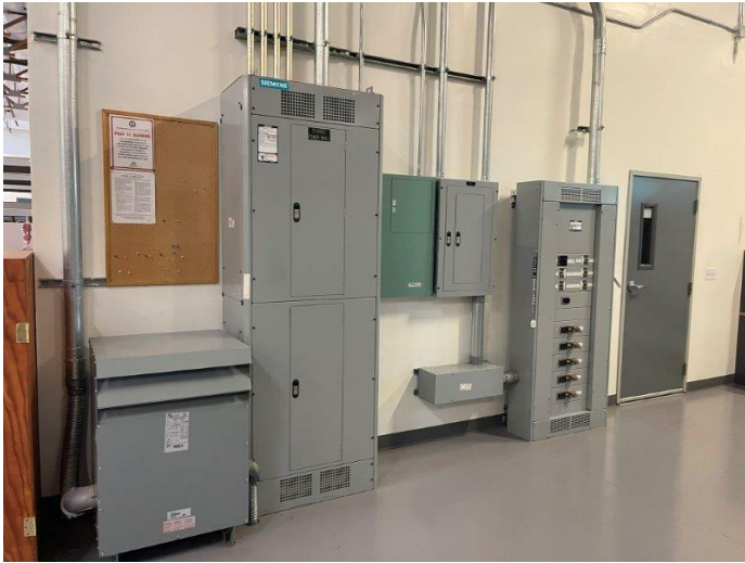
31. Warehouse electrical distribution system includes distribution transformer.
