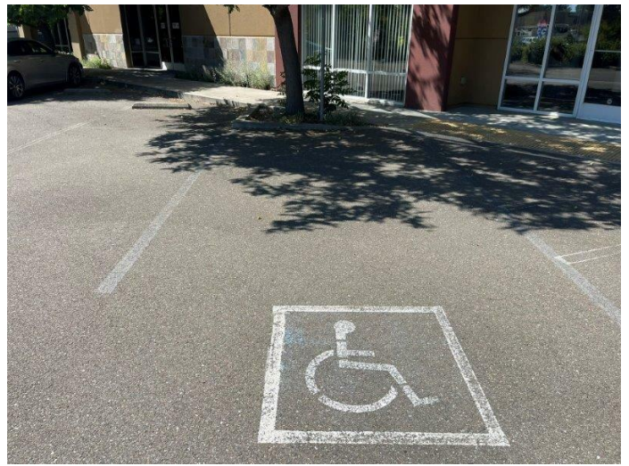
52. Designated ADA parking stall ground markings are faded.
