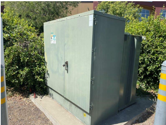
33. Eastern perimeter: one utility-owned pad-mounted transformer and one subgrade transformer noted.
