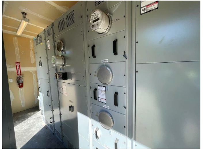
32. Main electrical distribution room (accessible from southern exterior door).
