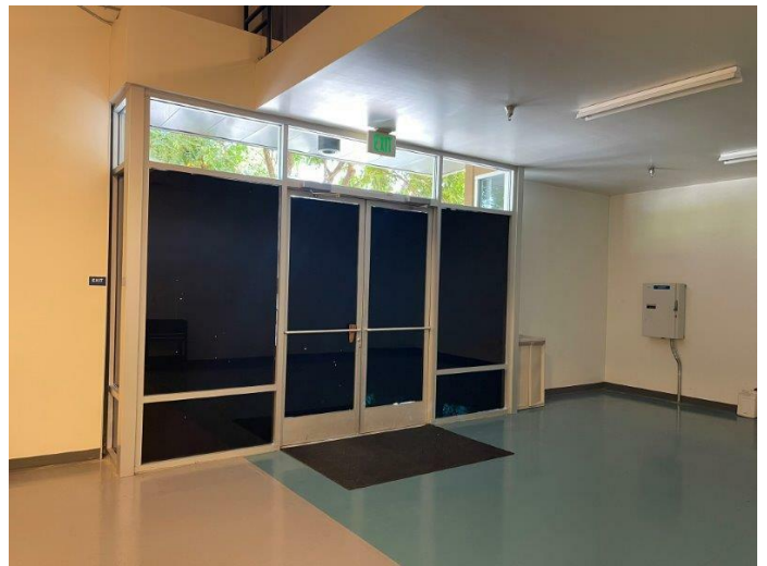
28. Entrance doors are double-hung units with full-height glazing in brushed aluminum storefront systems.
