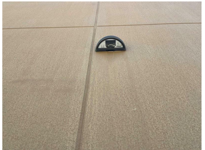
16. Exterior lighting includes facade-mounted LED wall packs along the northern, southern, and western sides.
