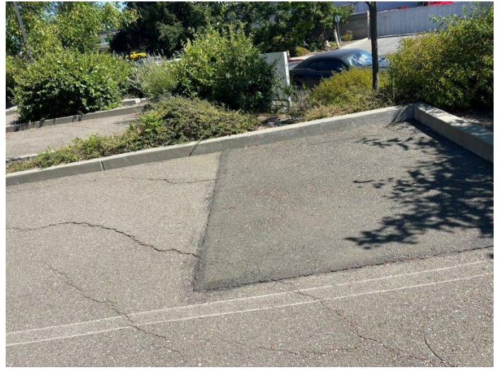
50. Linear cracking in asphalt paving and condition of stall striping.
