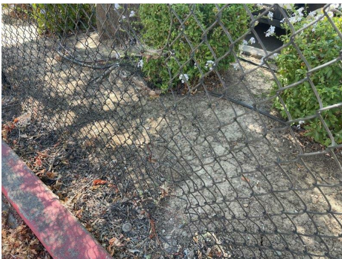
53. Southwestern parcel corner: chain-link fencing has been cut.
