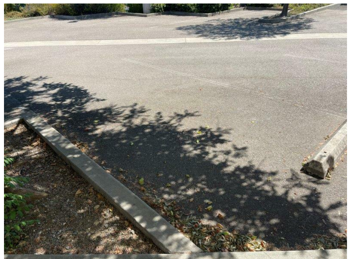
12. Asphalt paving: showing condition.
