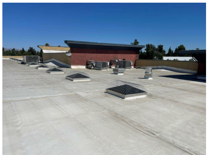
24. Skylights and HVAC equipment.
