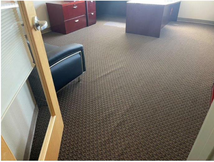
49. Mezzanine, office: carpeting is worn and warping.
