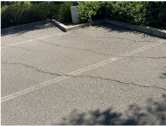
51. Linear cracking in asphalt paving and condition of stall striping.
