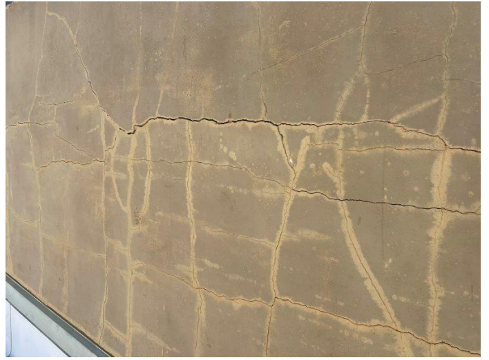
56. Rooftop, mezzanine penthouse: damaged stucco.
