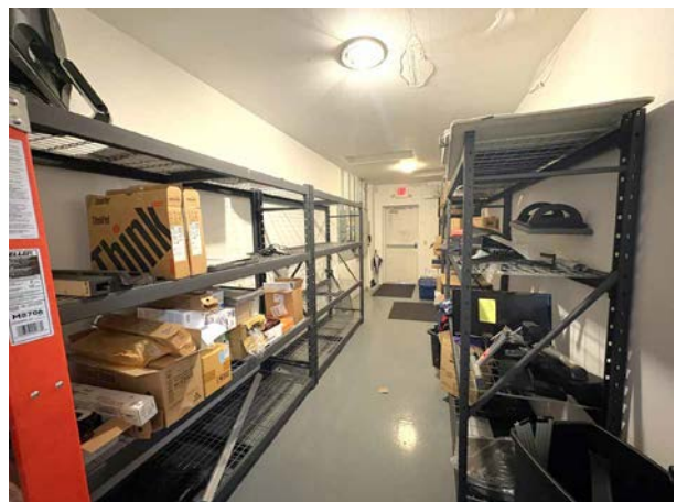
West Office - Mechanical Room
