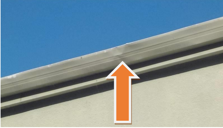
Item #19-Rain gutters-Across the rear of the building, some of the gutter material is dented
