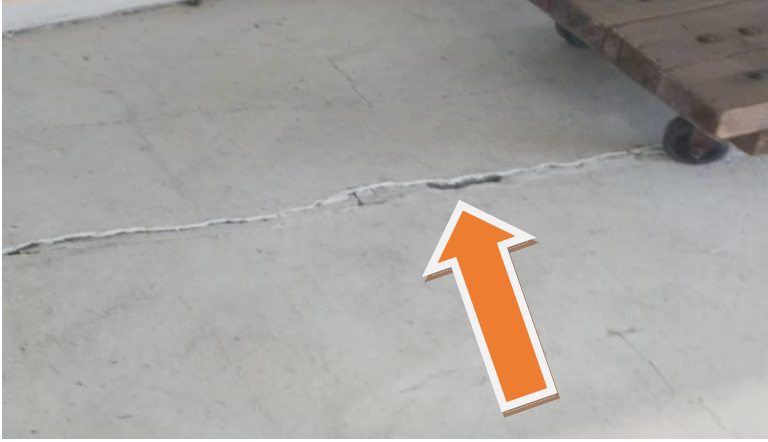
Item #270-Sea Green storage room, walls-At the entry door from the display room, there is a crack in the wall (may be associated with item #259)
