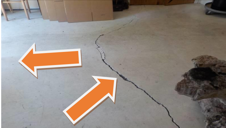
Item #259-Sea Green left side display room, floor-Toward the rear of the room, there are a few cracks, some wider than others/sloping floor
