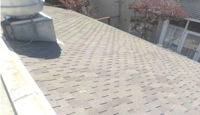
Item #29-Roof-The 50-year composite shingle roofing material is in good condition/below; over the end of unit G
