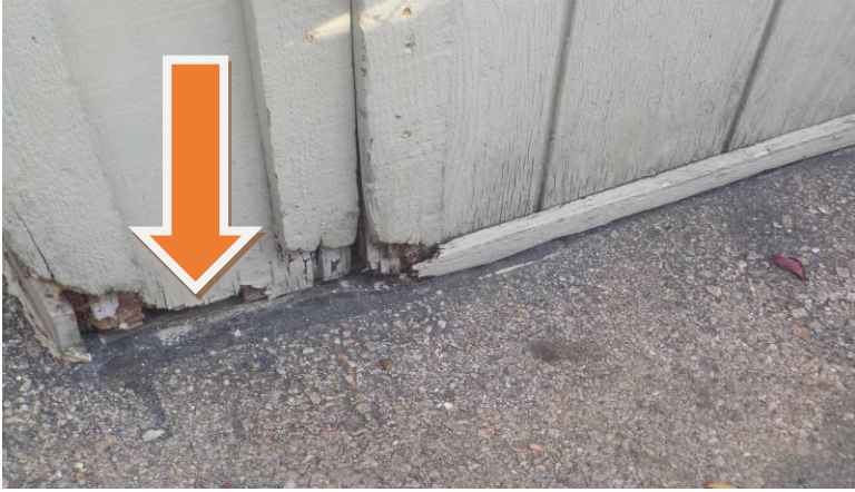
Item #23-Siding-At the storage area near the rear of Wild Ginger, some of the wood siding is damaged
