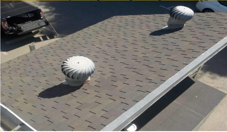
Item #29-Roof-The 50-year composite shingle roofing material is in good condition/below; over the front entry of units D and C
