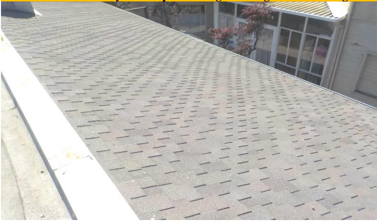
Item #29-Roof-The 50-year composite shingle roofing material is in good condition/below; over the end of unit G
