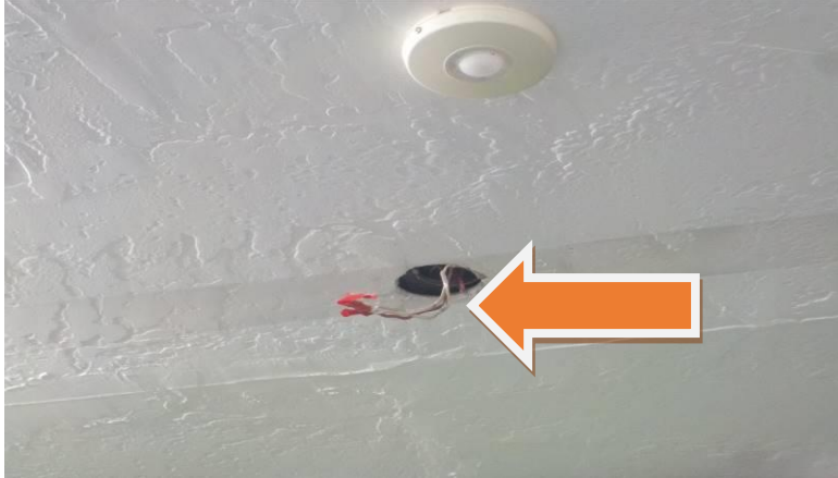
Item #221-Unit E, lighting-At the rear of the retail area/Smoke Shop, the light fixture has been removed/the termination of wiring is not safe
