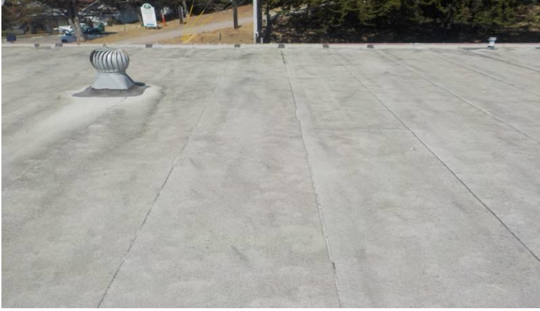
Item #29-Roof-The 'Torch' style roofing material is in fair condition/below; over the rear half of units A and F
