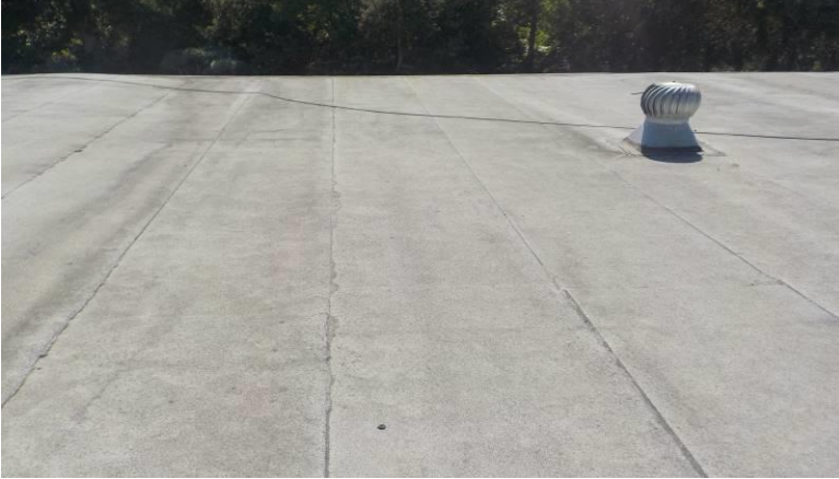
Item #29-Roof-The 'Torch' style roofing material is in fair condition/below; over the front half of unit A
