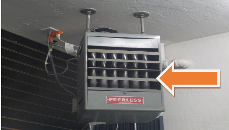
Item #224-Unit E, heat source-This heating unit in the Smoke Shop is not operating/thermostat is behind the cabinets/not accessible
