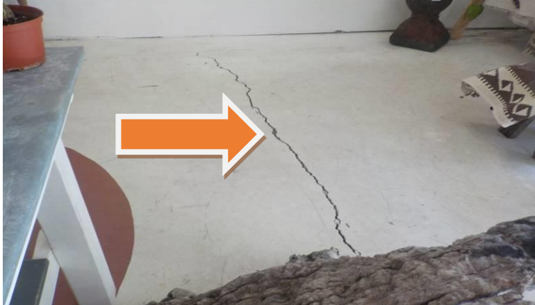
Item #259-Sea Green left side display room, floor-Toward the rear of the room, there are a few cracks, some wider than others/sloping floor
