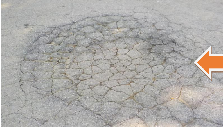
Item #0-Parking lot-At the back corner of the parking lot, there are a few areas where the asphalt is cracking and settling
