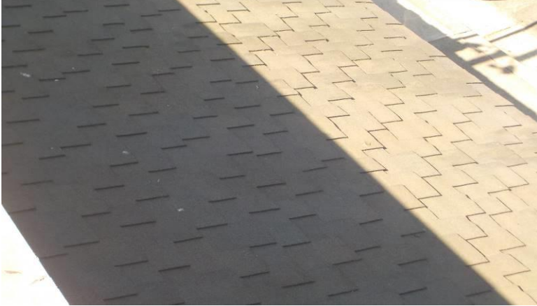
Item #29-Roof-The 50-year composite shingle roofing material is in good condition/below; over the front corner of unit G
