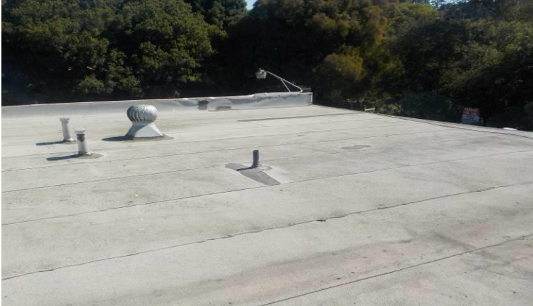
Item #29-Roof-The 'Torch' style roofing material is in fair condition/below; over unit C
