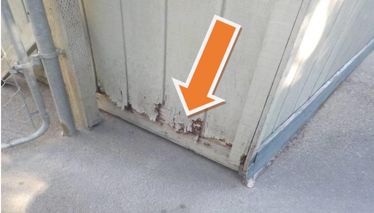
Item #23-Siding-At the fire sprinkler storage room on the side of Wild Ginger, some of the wood siding is damaged
