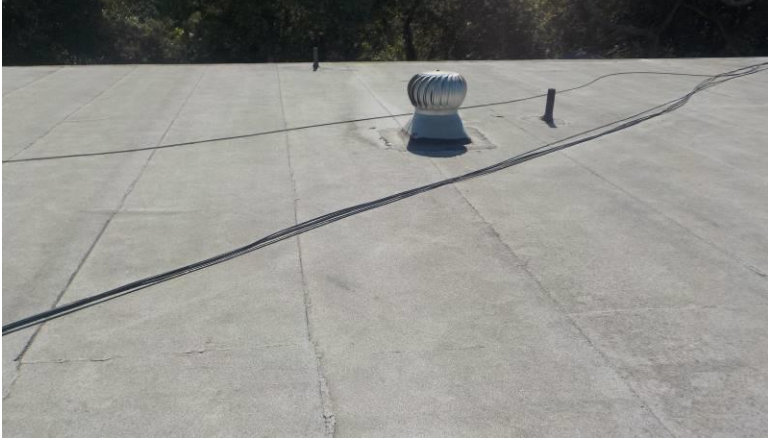
Item #29-Roof-The 'Torch' style roofing material is in fair condition/below; over the front half of unit G
