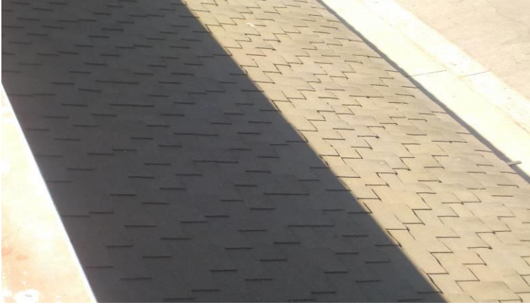
Item #29-Roof-The 50-year composite shingle roofing material is in good condition/below; over the front entry of unit G
