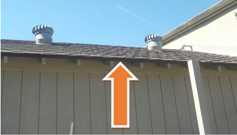
Item #19-Rain gutters-There are no rain gutters over the front and side edges of the roof/gutters are recommended
