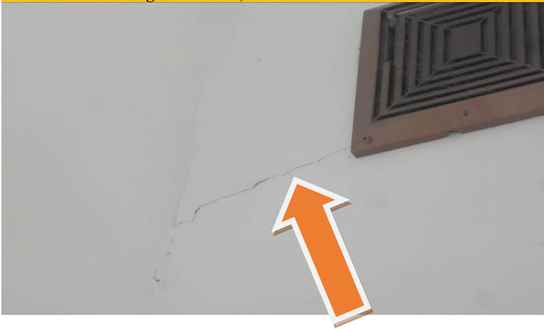
Item #159-Wild Ginger restroom, walls and door-The descending gap at the top of the door to door frame is probably due to the room slanting
