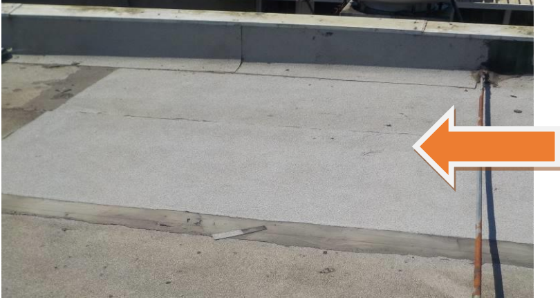
Item #29-Roof-The 'Torch' style roofing material is in fair condition/below; over unit D
