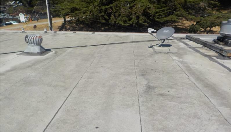
Item #29-Roof-The 'Torch' style roofing material is in fair condition/below; over the rear half of units B and E
