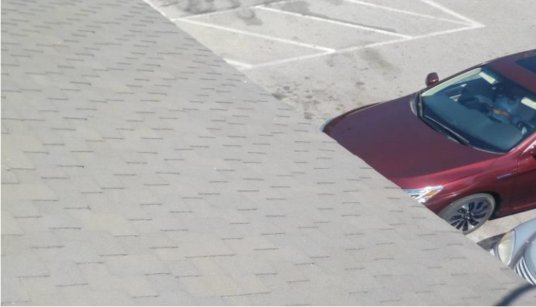
Item #29-Roof-The 50-year composite shingle roofing material is in good condition/below; over the front entry of units C and B
