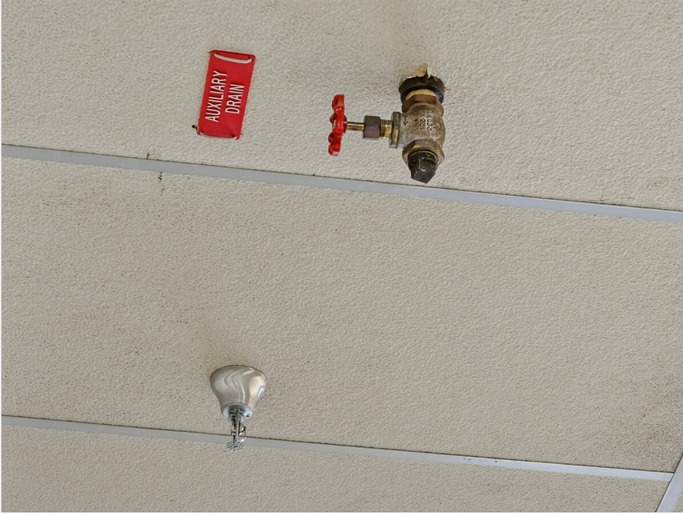
Sprinkler System on all levels
