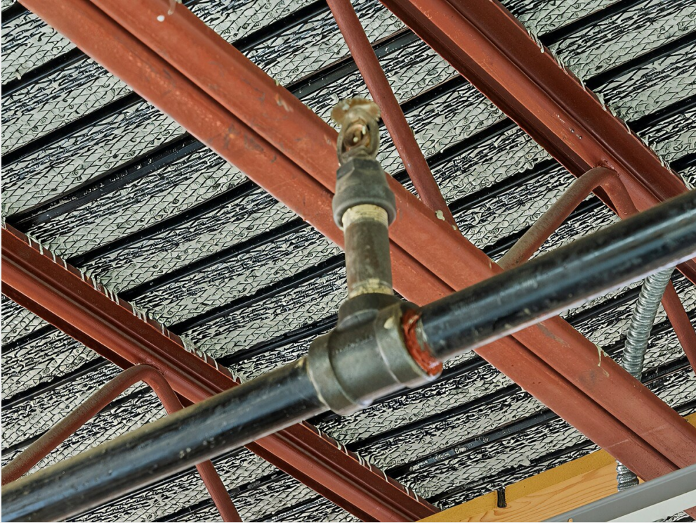
Sprinkler system on all levels
