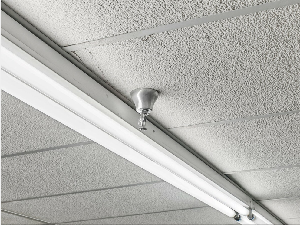
Sprinkler System on all levels
