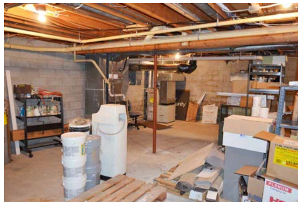
West Office - Lower Level Utility Room
