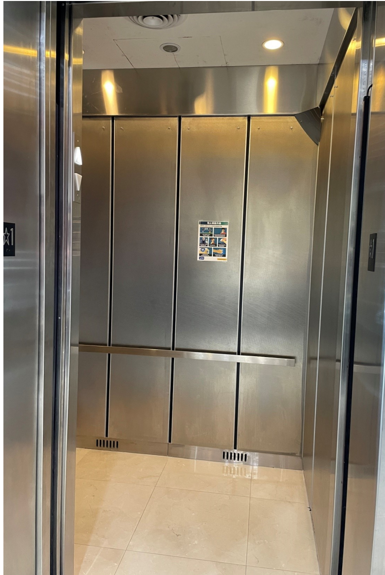
Passenger Elevator from Basement to 3rd Floor
