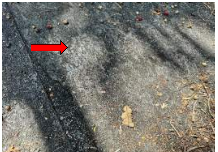
ROOF DAMAGE/EXPOSED FELT
