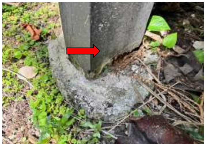
WOOD DECAYING FUNGI (WOOD ROT)
