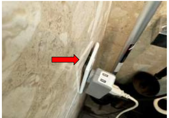
IMPROPERLY SEATED OUTLET
