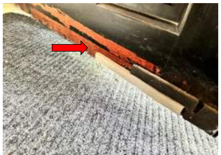
MISSING/DAMAGED WEATHER STRIP
