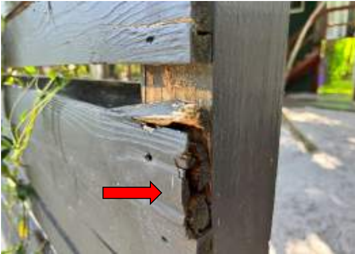
WOOD DECAYING FUNGI (WOOD ROT)
