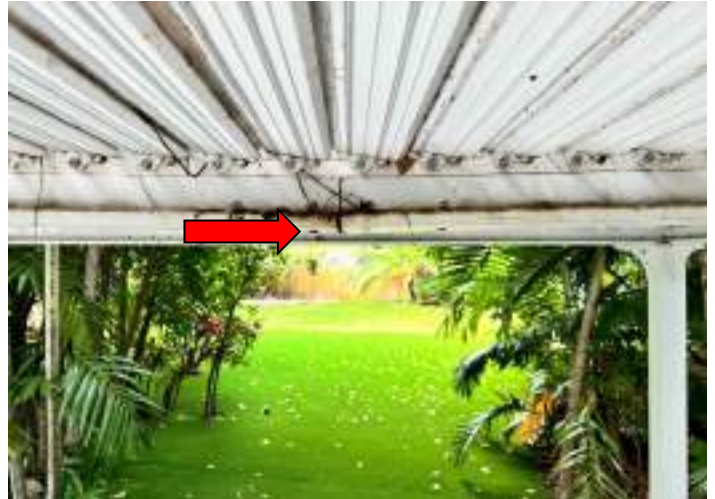
RUST/CORROSION - LOOSE JOINT
