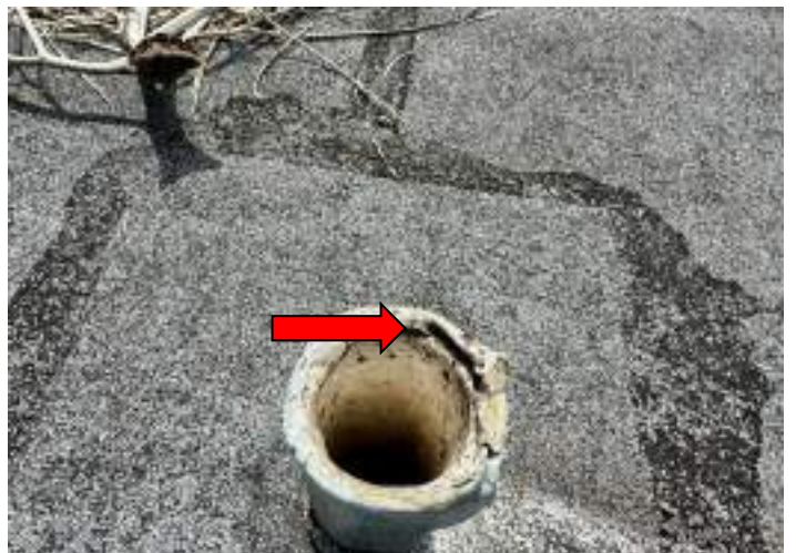
IMPROPERLY TERMINATED VENT PIPE
