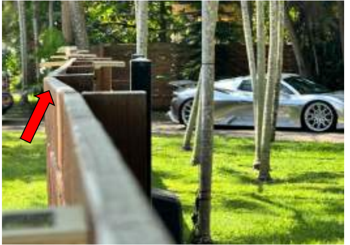
FENCE NOT ALIGNED
