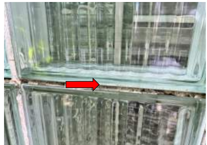
DAMAGED GLASS BLOCKS
