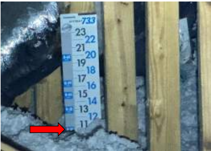
LOW INSULATION LEVEL
