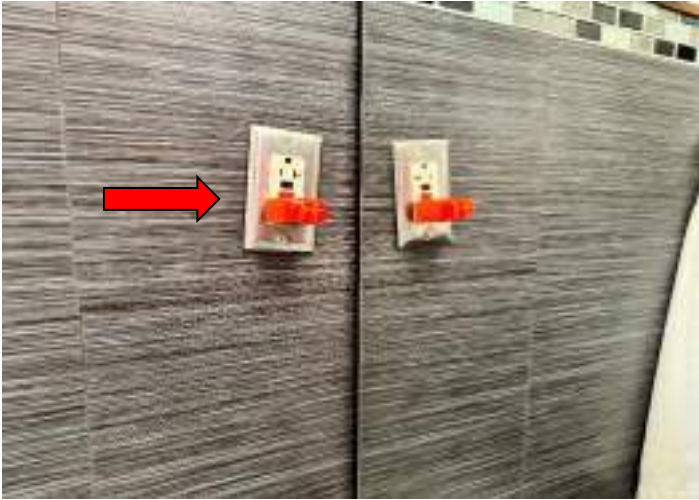
OUTLET NOT GFCI PROTECTED
