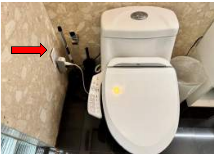
IMPROPERLY SEATED OUTLET
