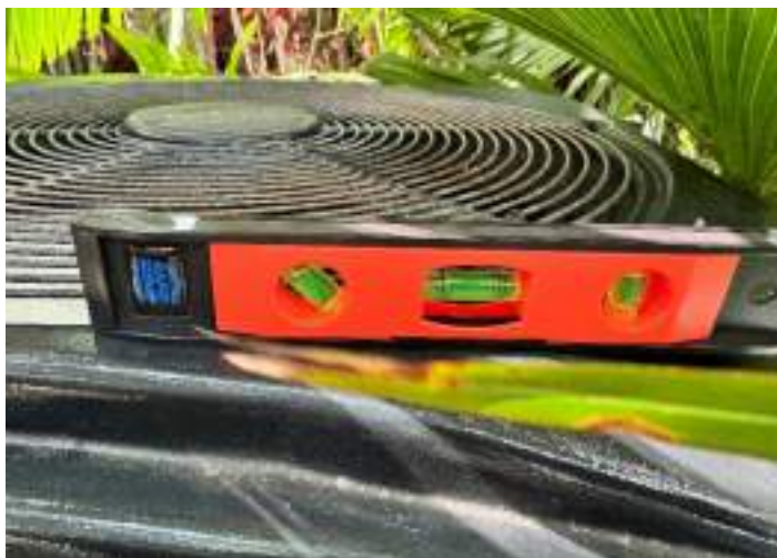
UNEVEN POOL HEATER
