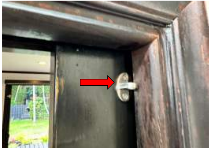
MASTER BATHROOM DOOR NOT FULLY OPEN
