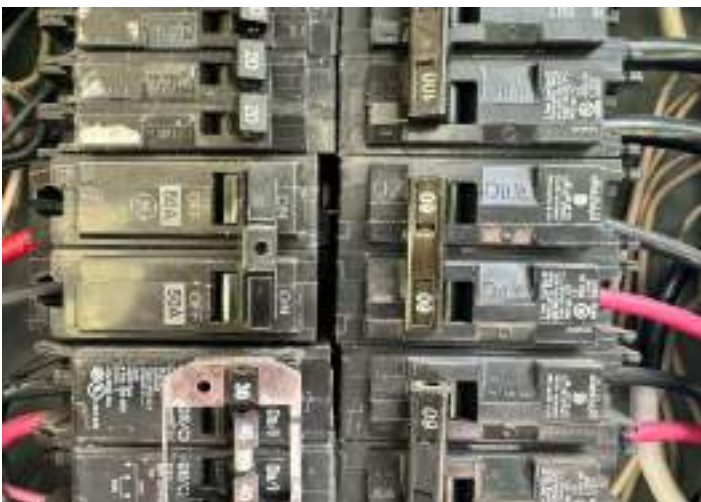
MISMATCHED CIRCUIT BREAKERS
