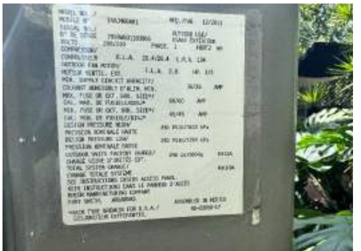
CONDENSING UNIT LABEL
