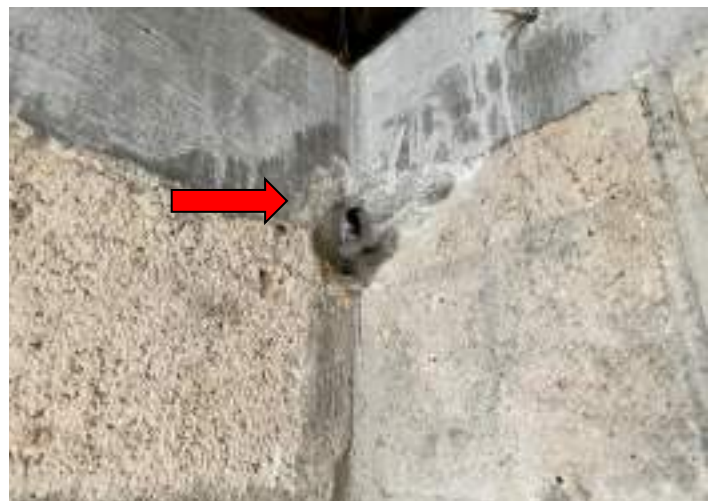
CHIPPED CONCRETE/ EXPOSED EMT CONDUIT
