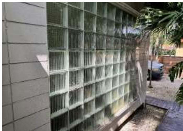
DAMAGED GLASS BLOCKS
