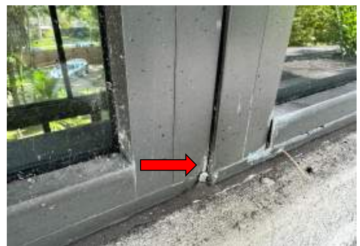
DETERIORATED CAULK/UNEVEN WINDOW TRIM
