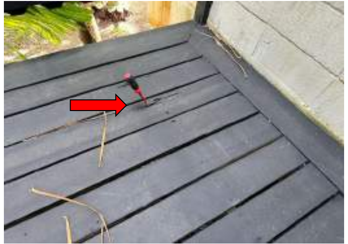
WOOD DECAYING FUNGI (WOOD ROT)
