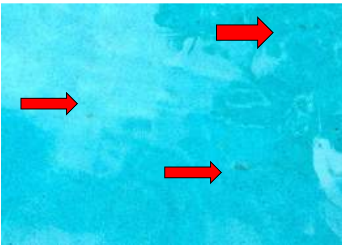
DAMAGED POOL SURFACE
