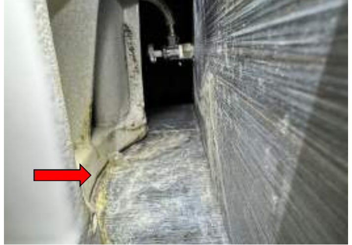
MOLD-LIKE SUBSTANCE/STAIN MARKS
