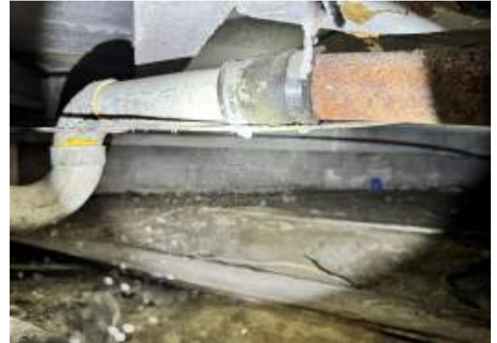
CAST IRON/PVC PIPE
