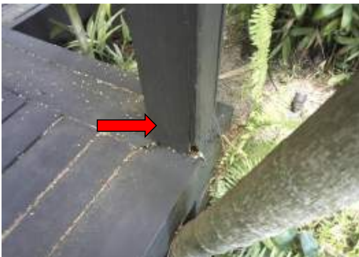
WOOD DECAYING FUNGI (WOOD ROT)
