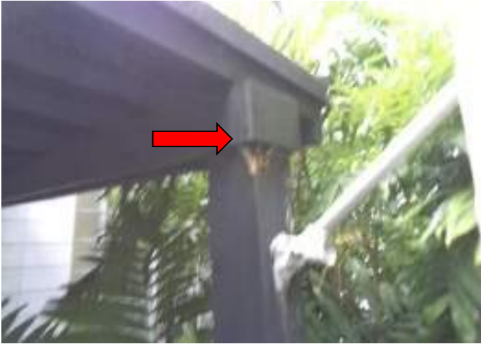
WOOD DECAYING FUNGI (WOOD ROT)
