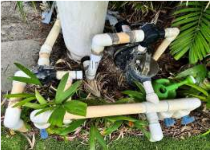
POOL PIPES NOT LABELED
