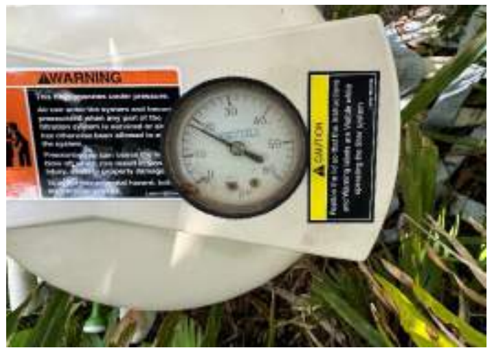
POOL FILTER GAUGE
