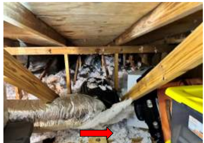
LOW INSULATION LEVEL
