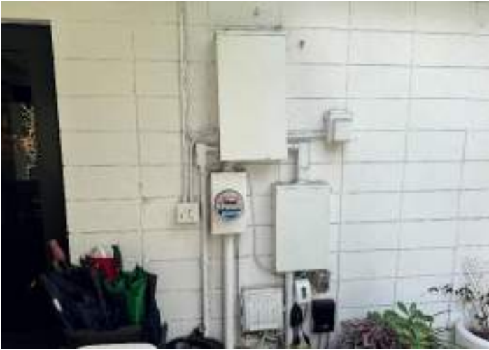
METER MAIN/MAIN DISCONNECTS
