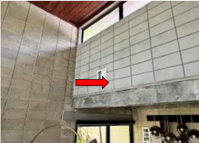
DAMAGED/CRACKED CONCRETE BLOCK
