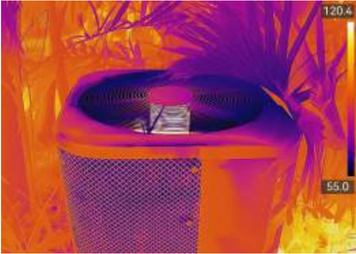
POOL HEATER OPERATIONAL
