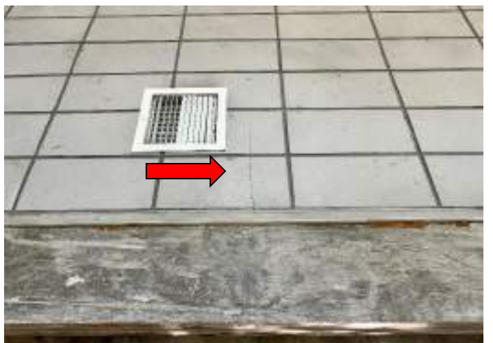
DAMAGED/CRACKED CONCRETE BLOCK
