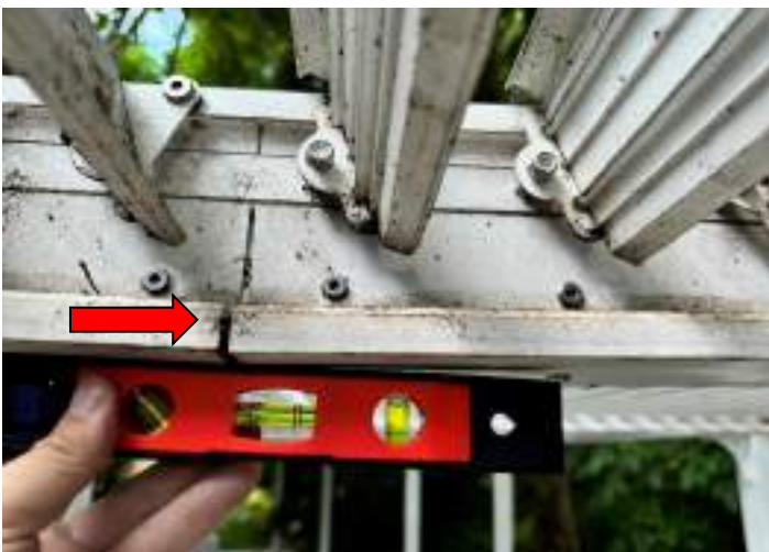
RUST/CORROSION - LOOSE JOINT
