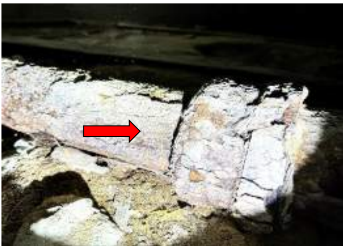
DETERIORATED CAST IRON PIPE
