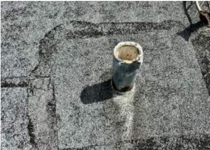
IMPROPERLY TERMINATED VENT PIPE
