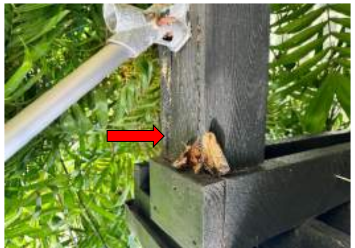
WOOD DECAYING FUNGI (WOOD ROT)
