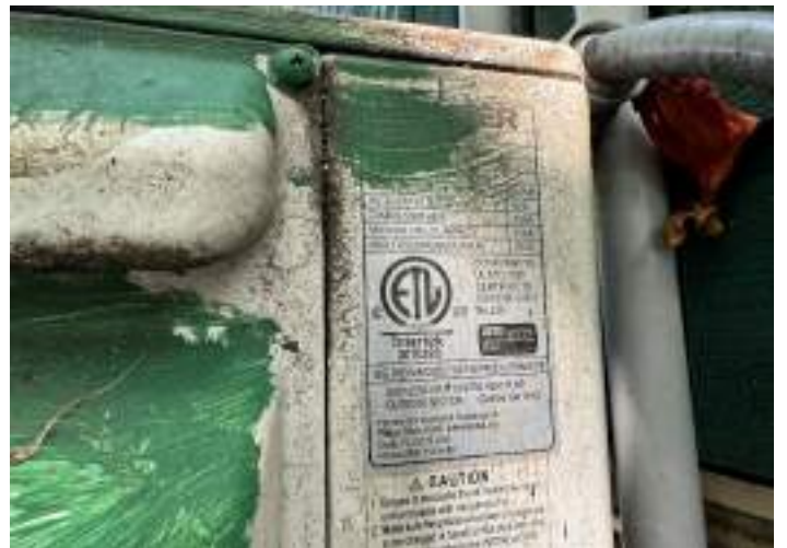
CONDENSING UNIT LABEL
