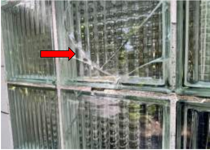
DAMAGED GLASS BLOCKS
