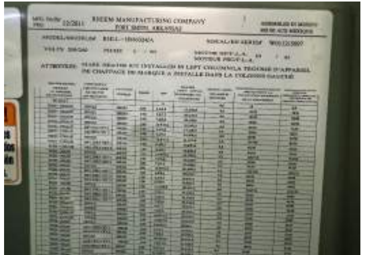
AIR HANDLER LABEL
