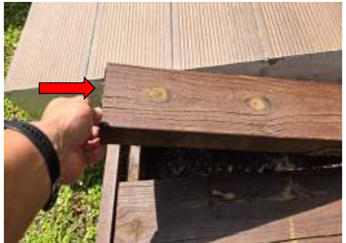
LOOSE WOODEN PLANKS
