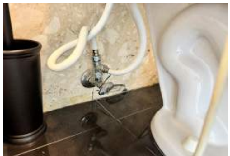
TOILET SHUT OFF VALVE
