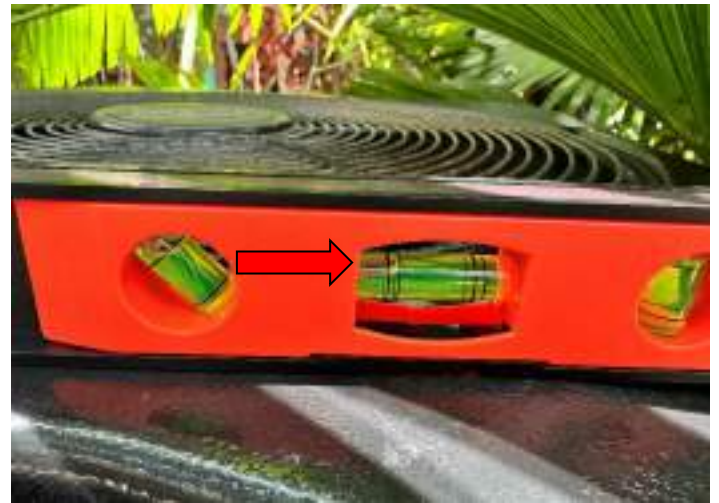
UNEVEN POOL HEATER
