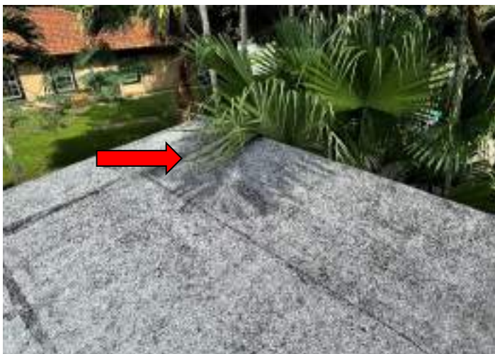
LEAVES, TREE BRANCHES TOUCHING ROOF SURFACE
