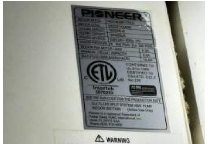
AIR HANDLER LABEL
