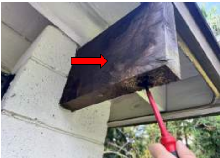
WOOD DECAYING FUNGI (WOOD ROT)
