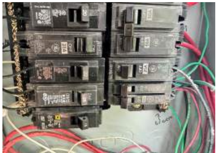
MISMATCHED CIRCUIT BREAKERS
