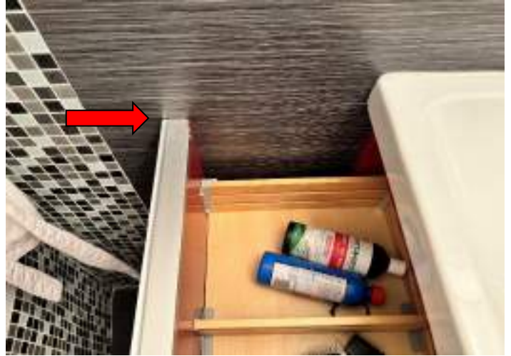
IMPROPERLY INSTALLED VANITY CABINET
