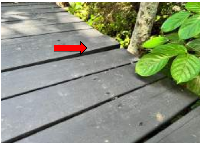
LOOSE WOODEN PLANKS
