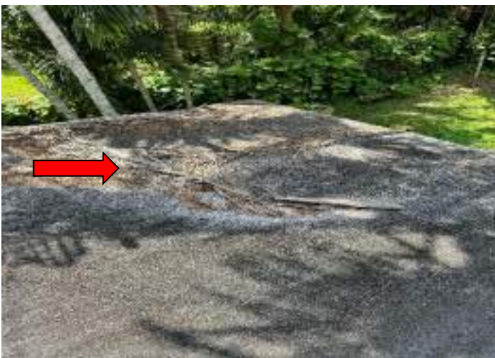
ROOF DAMAGE/EXPOSED FELT
