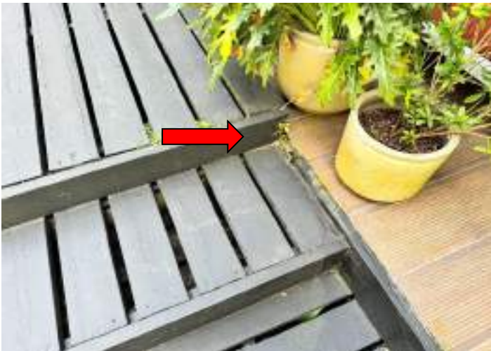
WOOD DECAYING FUNGI (WOOD ROT)
