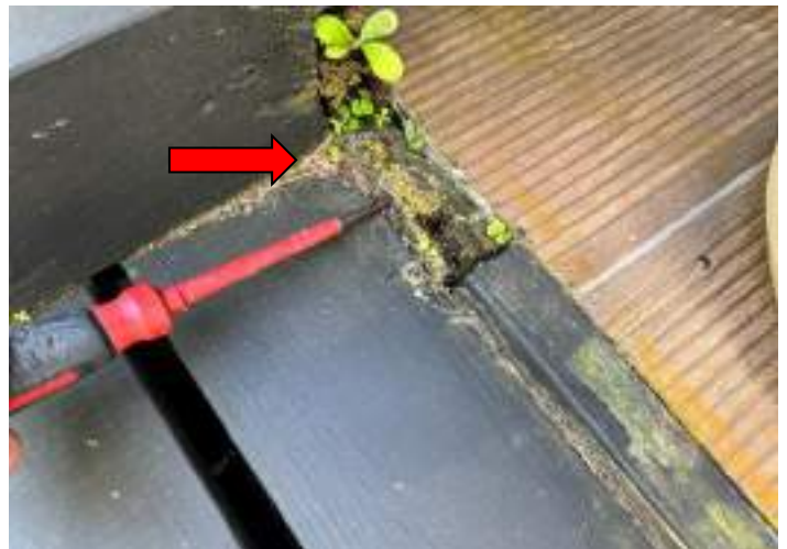
WOOD DECAYING FUNGI (WOOD ROT)
