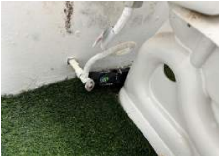
TOILET SHUT OFF VALVE
