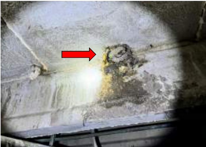
TERMINATED CAST IRON PIPE
