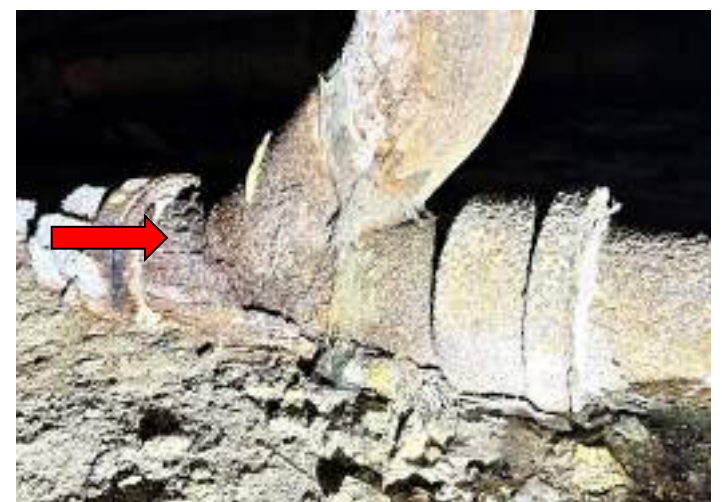
DETERIORATED CAST IRON PIPE
