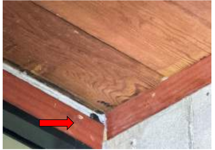
LOOSE CROWN MOLDING
