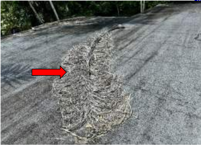
LEAVES, TREE BRANCHES TOUCHING ROOF SURFACE
