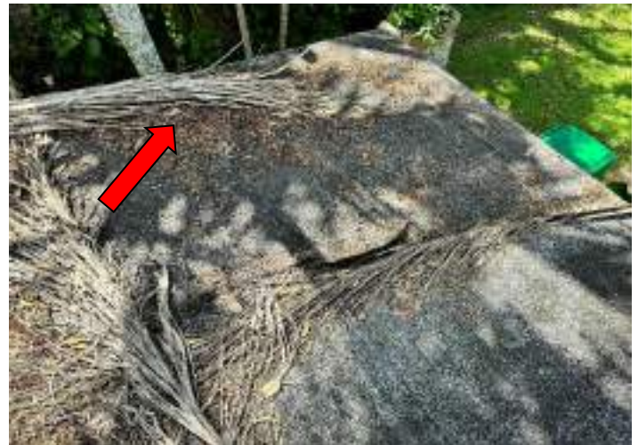
LEAVES, TREE BRANCHES TOUCHING ROOF SURFACE
