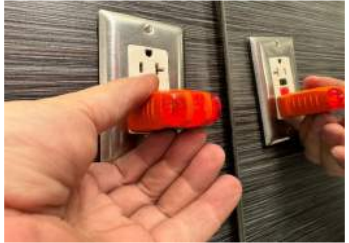
OUTLET NOT GFCI PROTECTED
