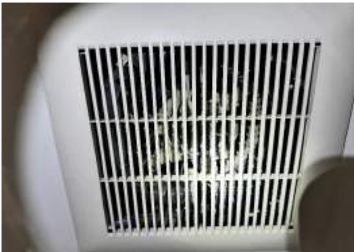
EXCESSIVE AMOUNT OF DUST
