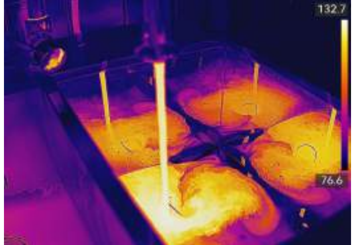
EVIDENCE OF HOT WATER 132.7 F
