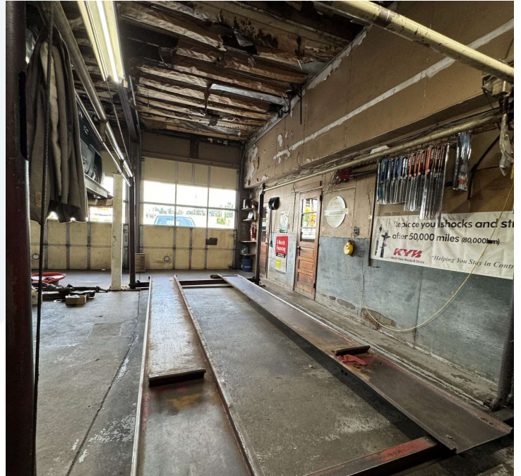
Main Lift Area - Lift 1
