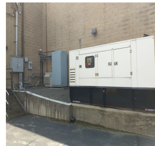
125 KVA diesel Generator
