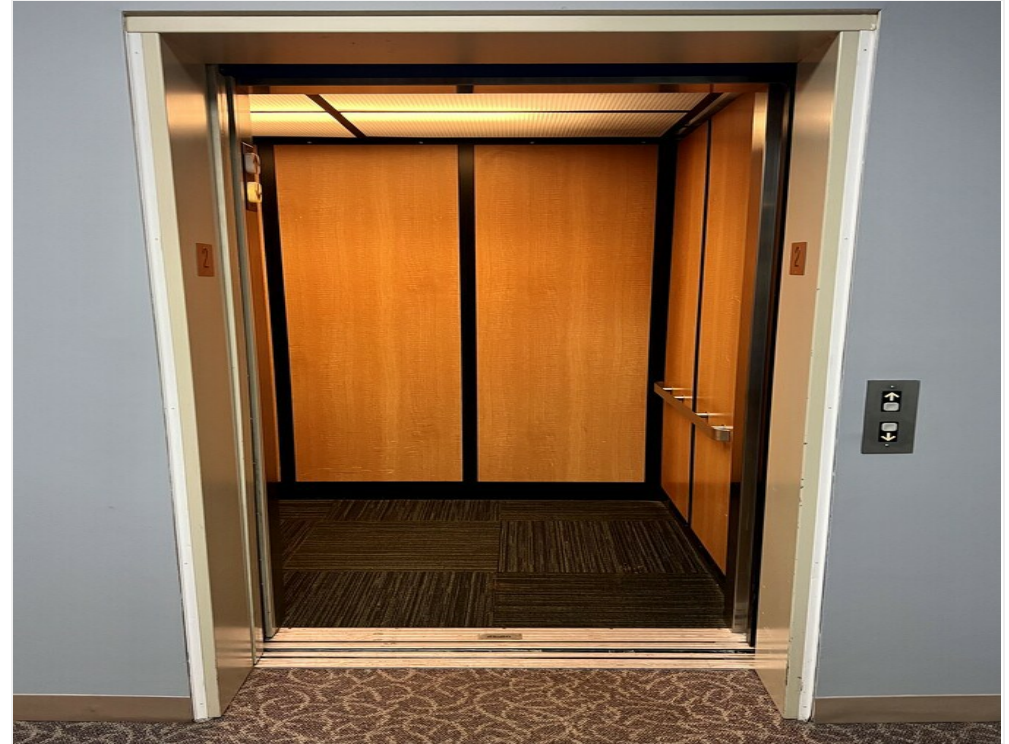
One of Two Elevators
