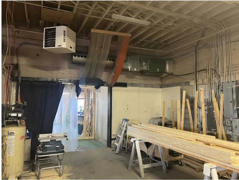
Interior bay with electrical meters – Workshop Level
