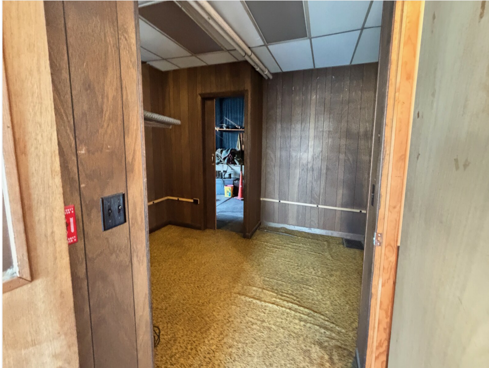
1st Fl - Office A-Side from Storefront A - with Door to Garage (c)
