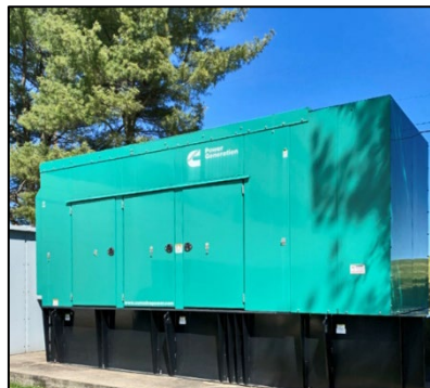
FULL BUILDING BACK-UP GENERATOR
