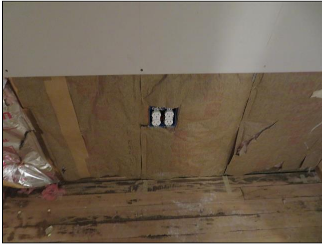
4.15.A Item 2(Picture) Utility room
