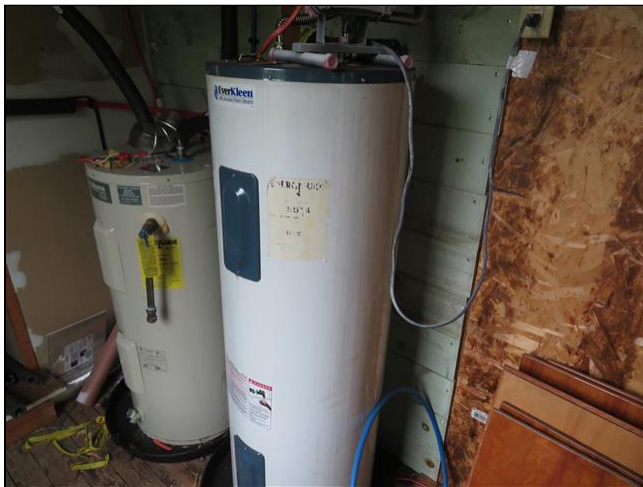
4.9.A Item 1(Picture) Utility room
