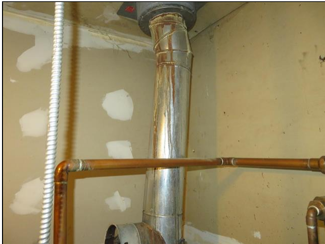
4.26.A Item 1(Picture) Utility room
