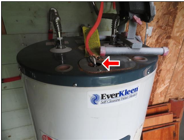
7.3 Item 2(Picture) Utility room
