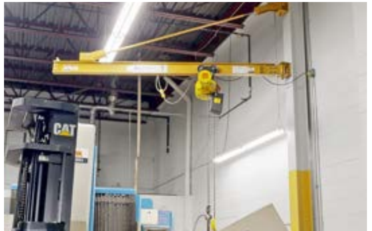
1-Ton Jib Crane - ±10'0" Under Hook (Bay 2)
