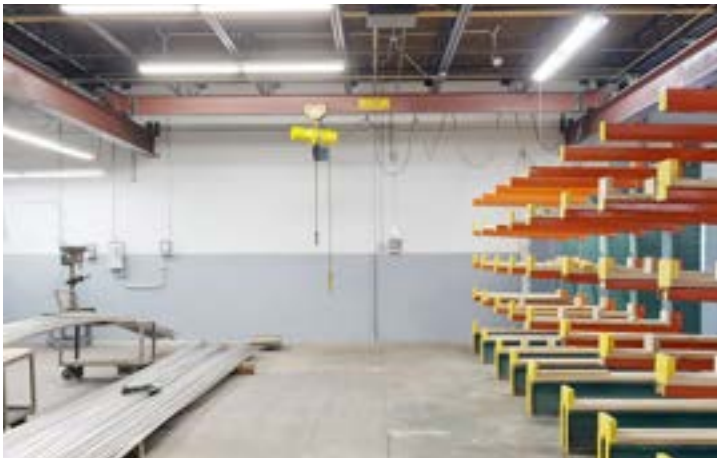
1-Ton Bridge Crane ±21'W x 32'L Rail System - ±8'2" Under Hook (Bay 1)
