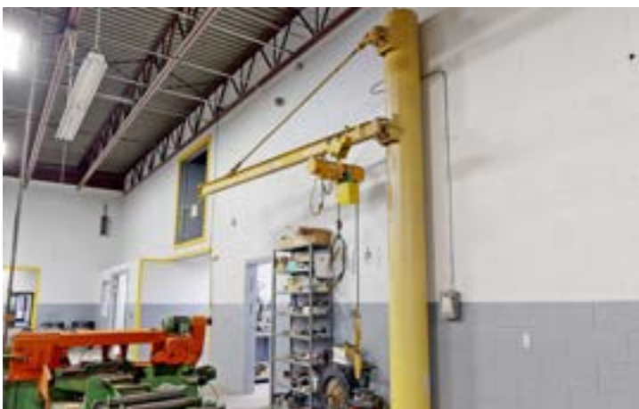
1-Ton Jib Crane - ±7'3" Under Hook (Bay 2)
