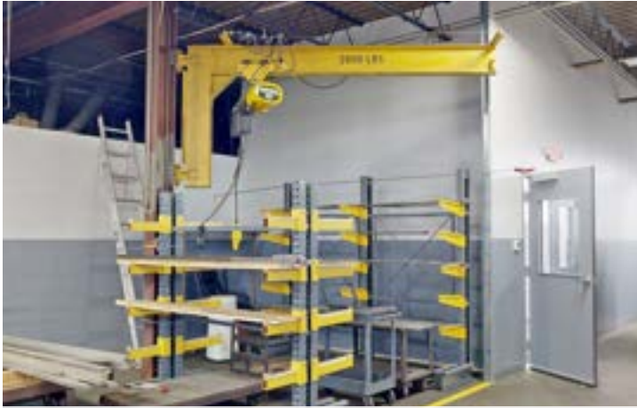
1-Ton Jib Crane - ±7'4" Under Hook (Bay 1)
