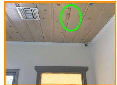
Example - Moisture Stain
