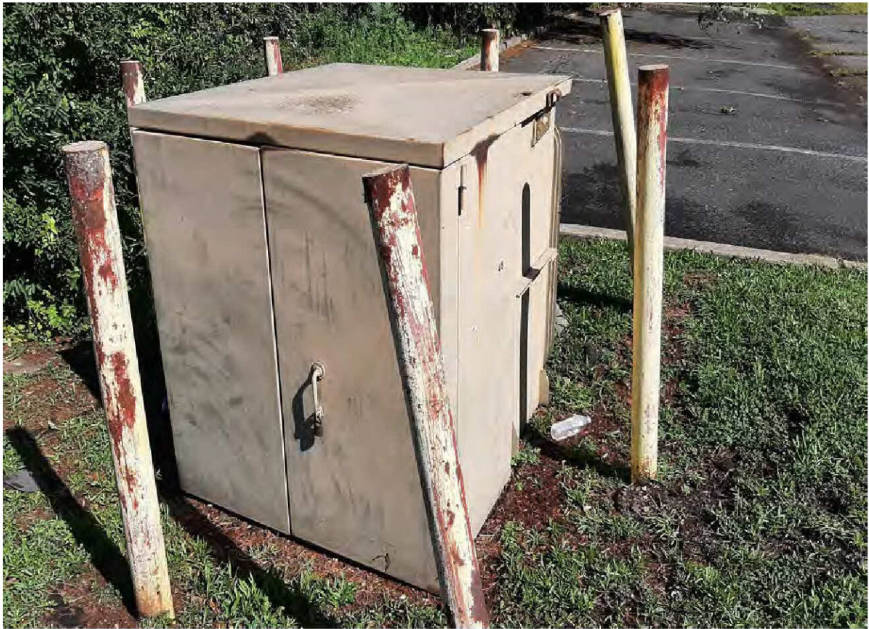
5. View of the pad-mounted transformer.
