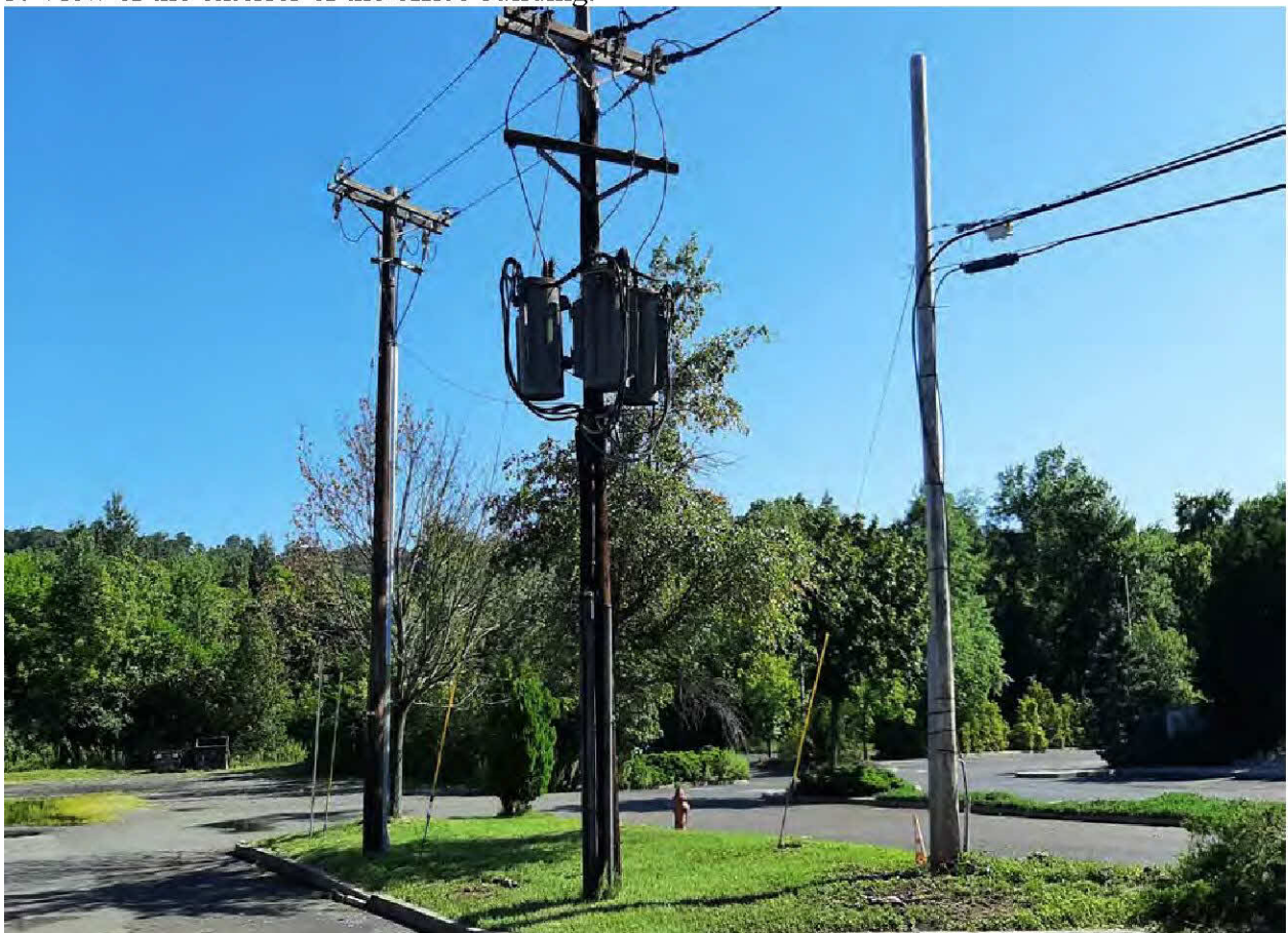
4. View of the pole-mounted transformers.
