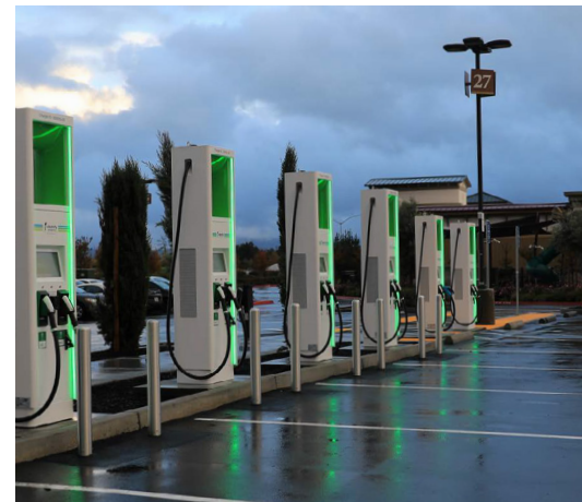
Electric Car Charging Stations
