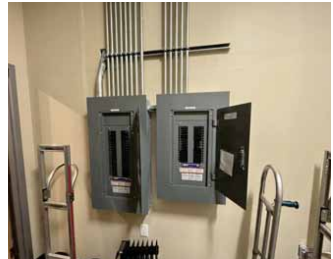
3463 - 2 Separate Electrical Panels
