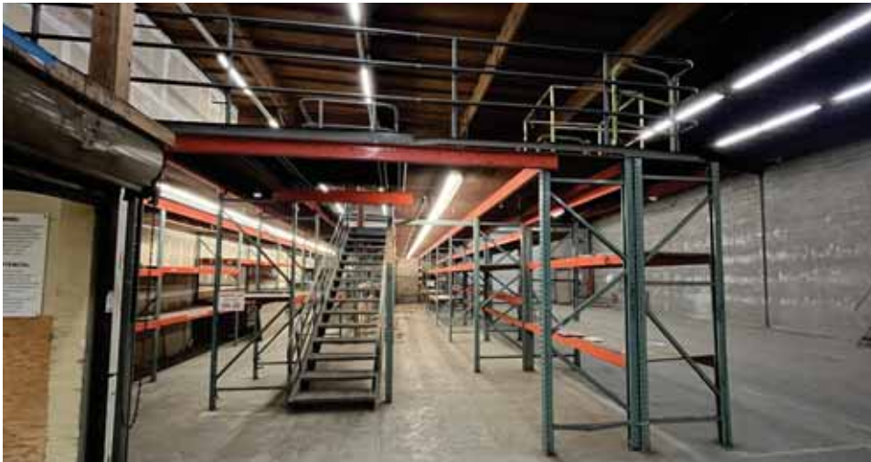
Mezzanine Steel Rack Storage System
