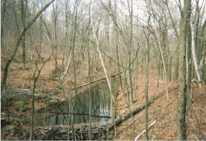
Existing Power Canal – Overgrown with small trees
