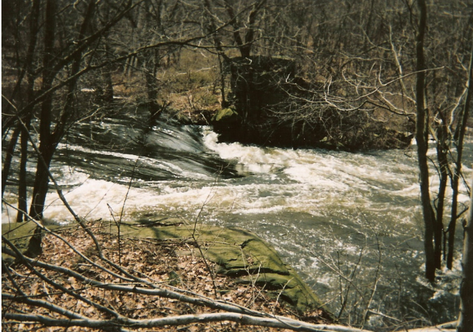
Breach on Upper Dam – 4-4-05 Spring Flows
