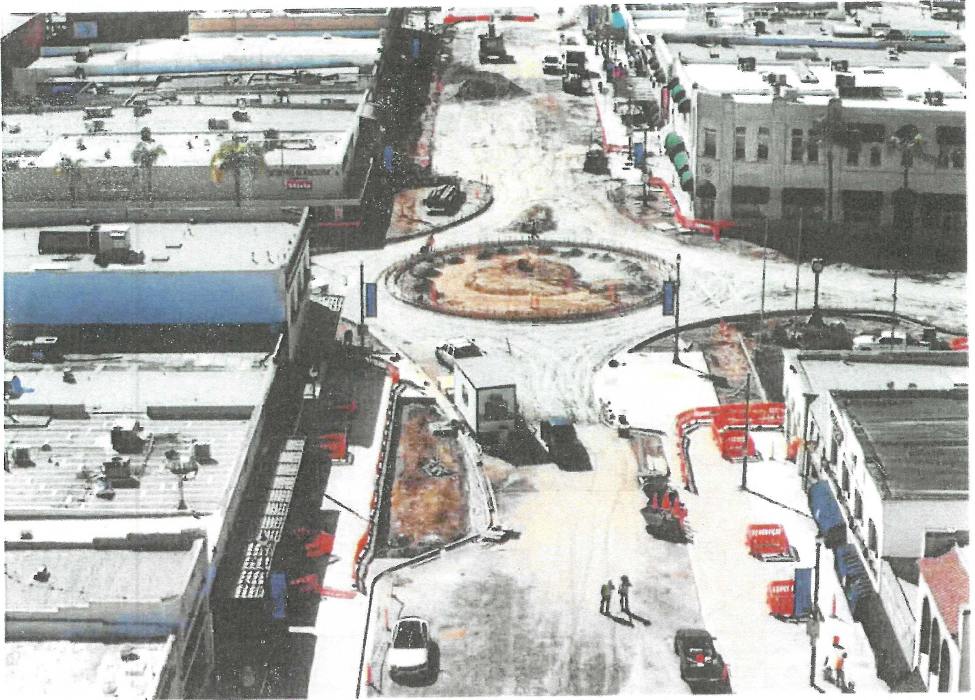
A drone photo shows a roundabout under construction on Broadway and Grand Avenue and other work being conducted as part of Escondido's Grand Avenue Vision Project. (Meg McLaughlin / The San
