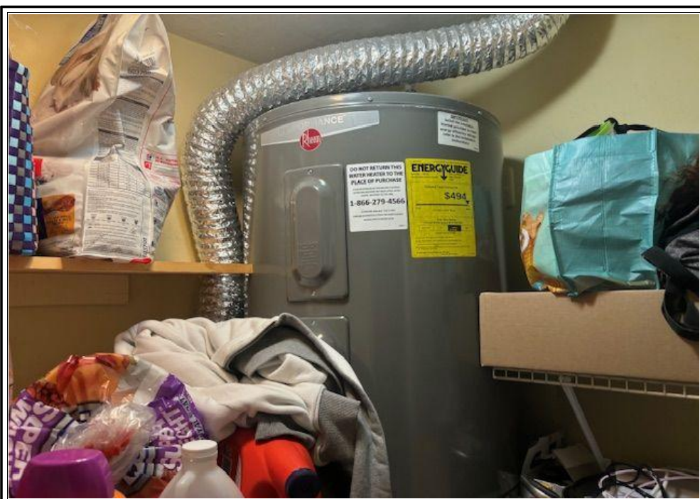
WATER HEATER UNIT B
