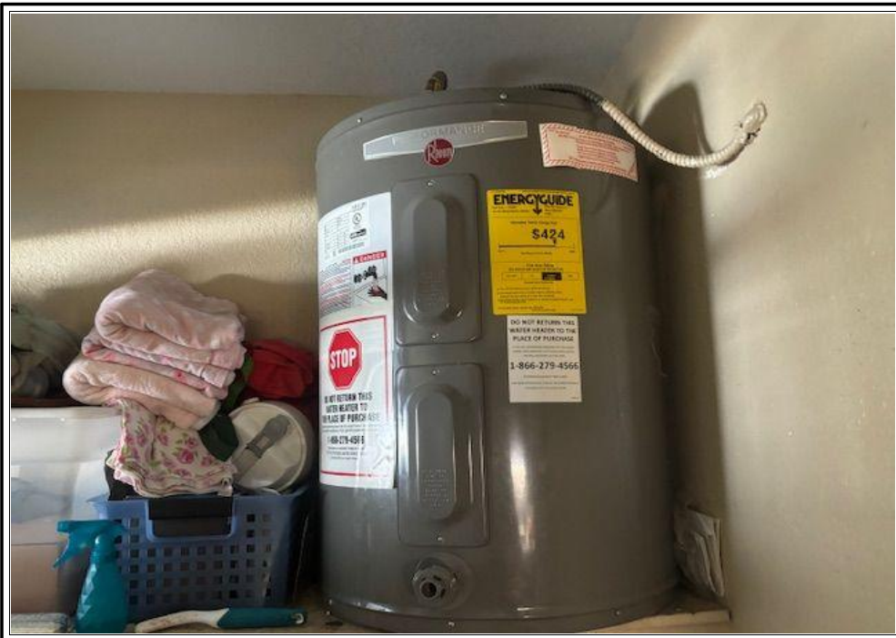
WATER HEATER UNIT A
