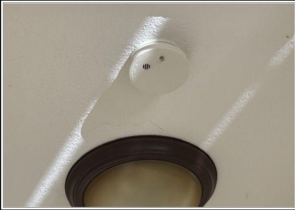
SMOKE DETECTOR UNIT A
