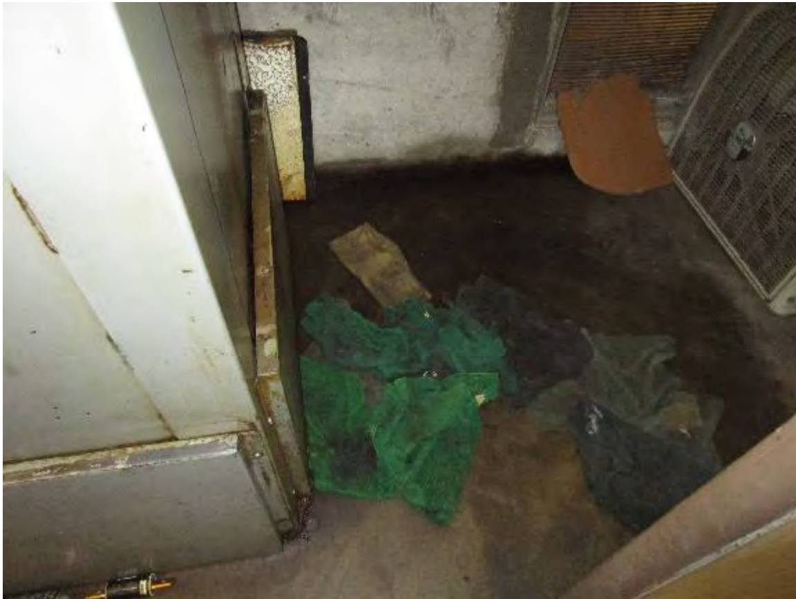
Passenger elevator equipment room showing new spill
