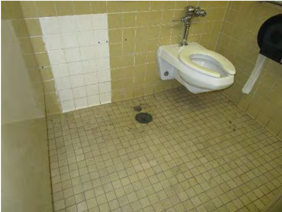
Basement restroom with floor drain
