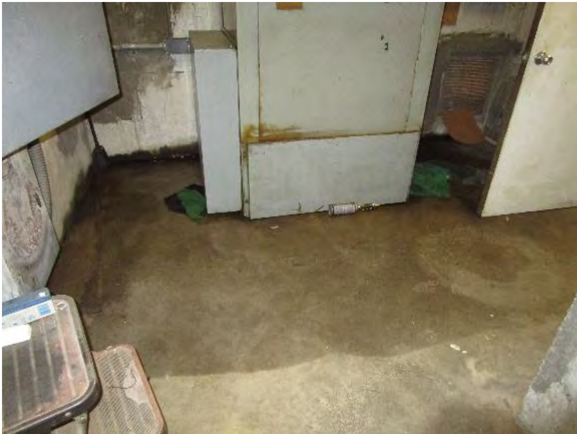
Passenger elevator equipment room showing former spill
