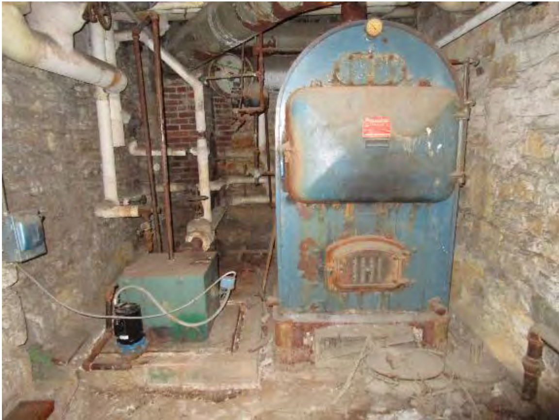
Basement-secondary boiler room
