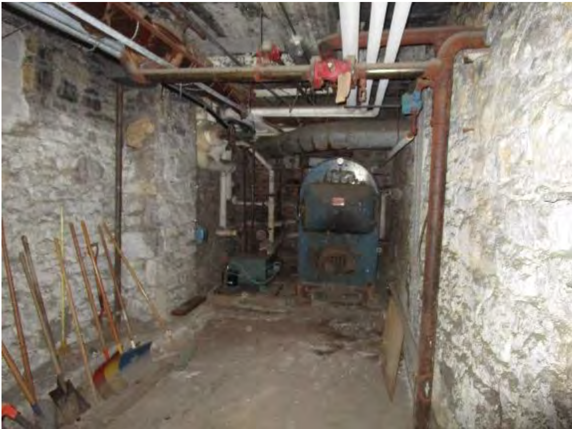
Basement-secondary boiler room
