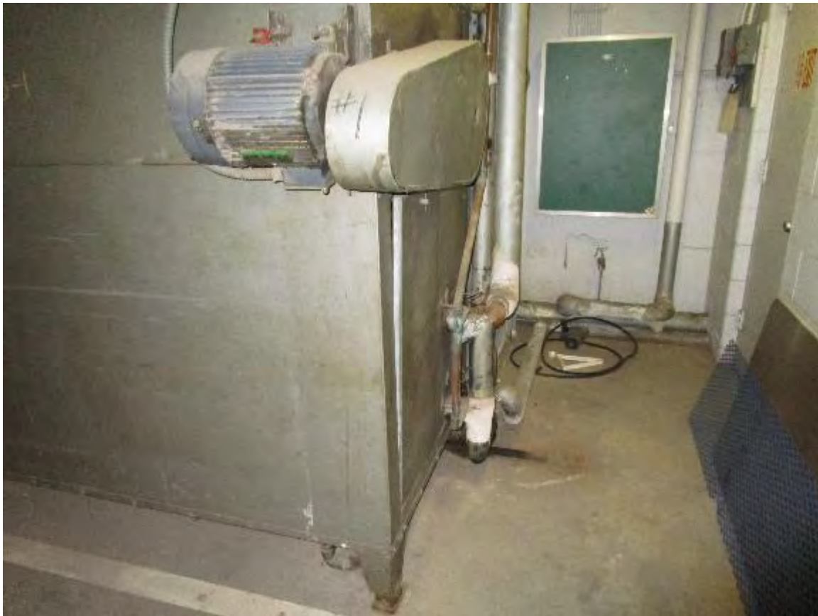
Basement air handler with floor drain
