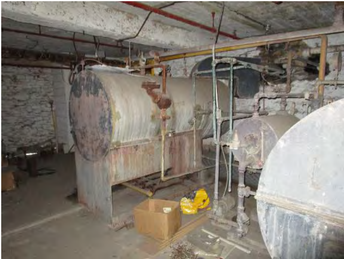
Basement-original boiler room
