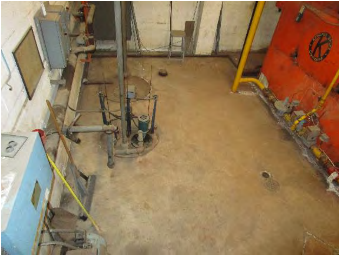
Basement-current boiler system showing floor drains and sump pump
