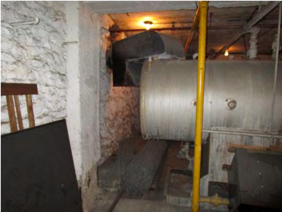
Basement-original boiler room
