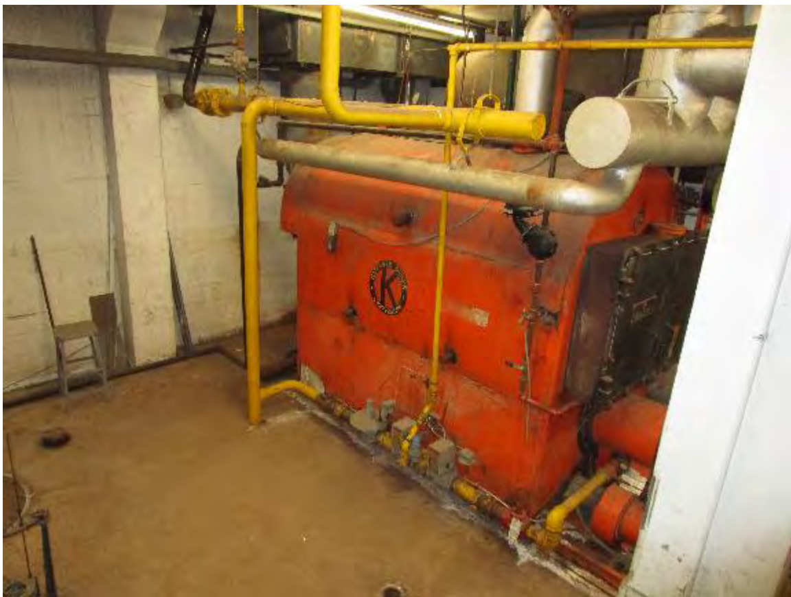
Basement-current boiler system
