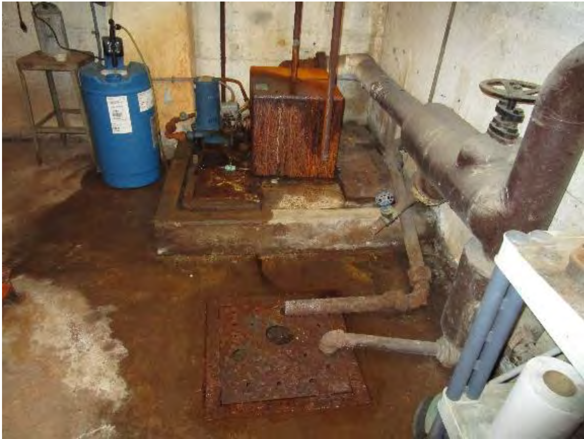
Basement-current boiler system
