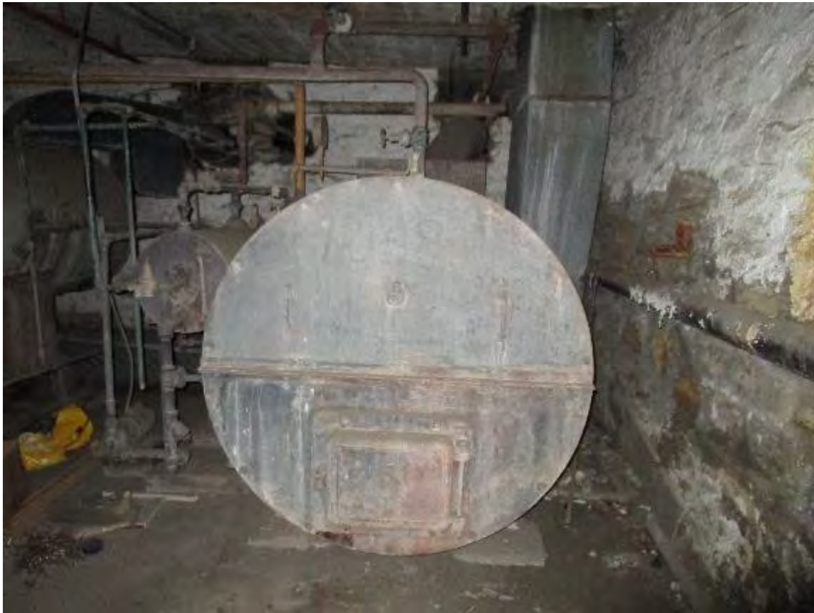
Basement-original boiler room
