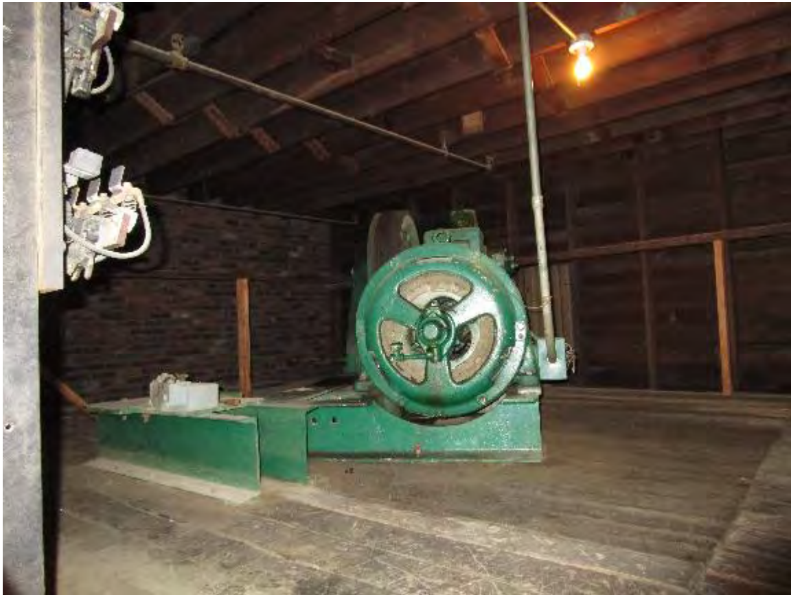
Penthouse elevator equipment room
