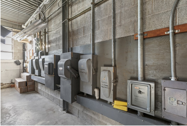
Heavy Power—400 Amp, 3 Phase
