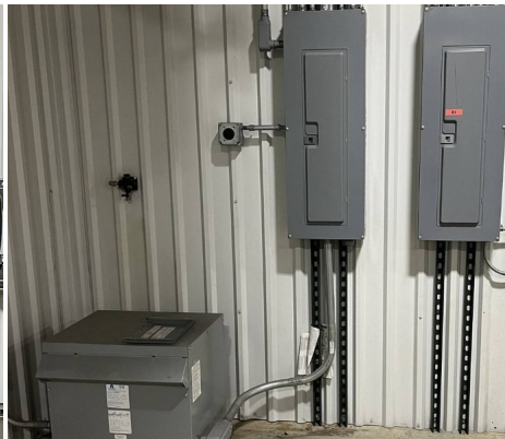
TRANSFORMER &amp; PANELS
