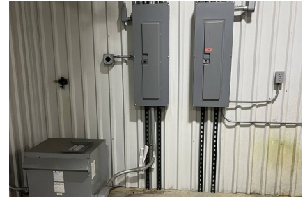
TRANSFORMER &amp; PANELS
