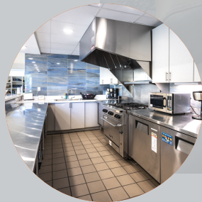
Full Commercial Kitchen
