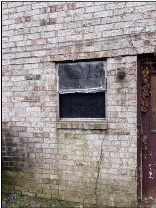
131. The window will cause loss of energy...
