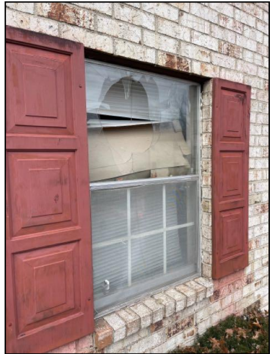
136. The window will cause loss of energy...
