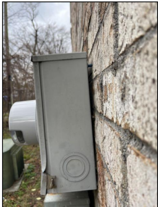
11. Electric panels, meter boxes, junction...
