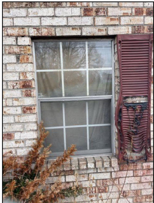
134. The window will cause loss of energy...
