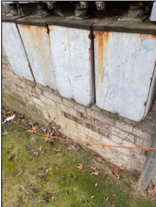
6. Electric panels, meter boxes, junction...
