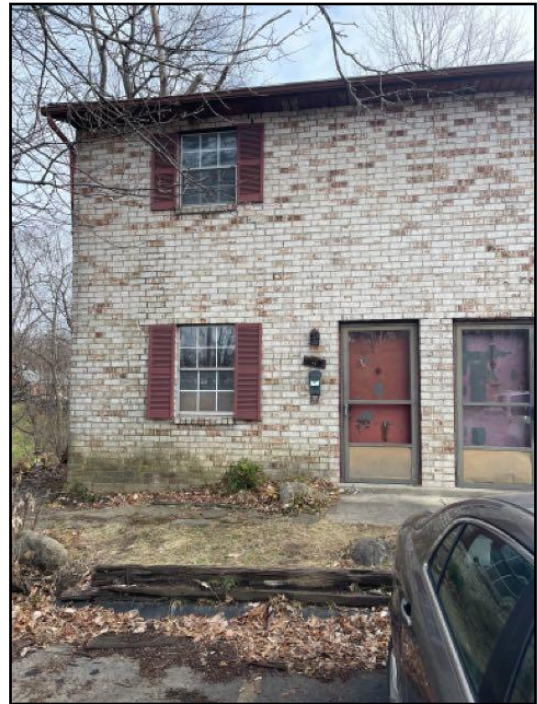
89. Fire damage was found. Consult the owner fo...
