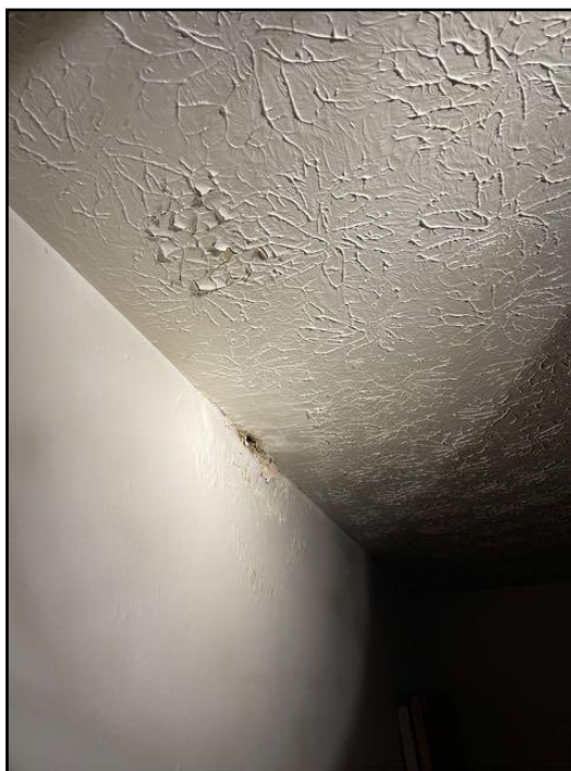
83. Water damage was found at this location....
