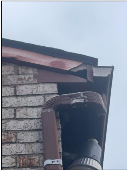
112. Siding has minor damage. Any opening should...
