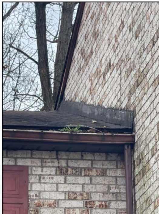
69. Not regletted into the masonry wall
