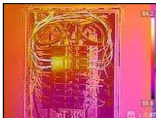
20. Infrared camera displays a thermal anomaly....
