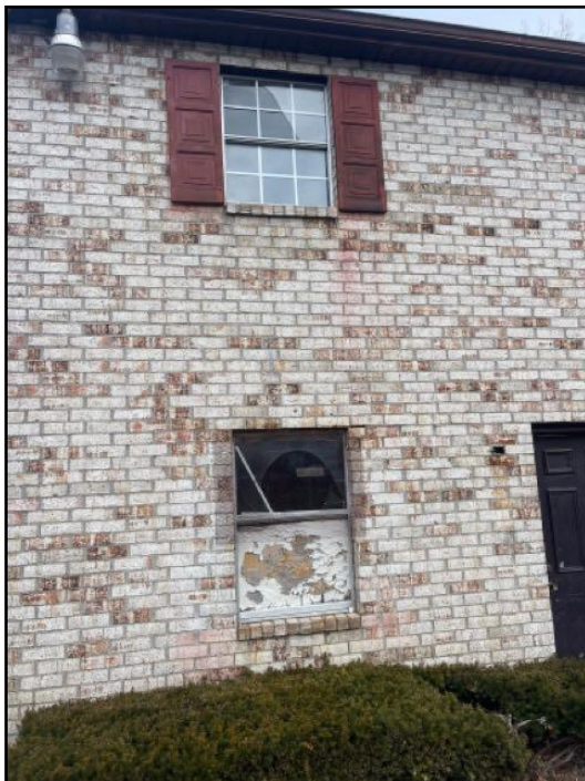
133. The window will cause loss of energy...
