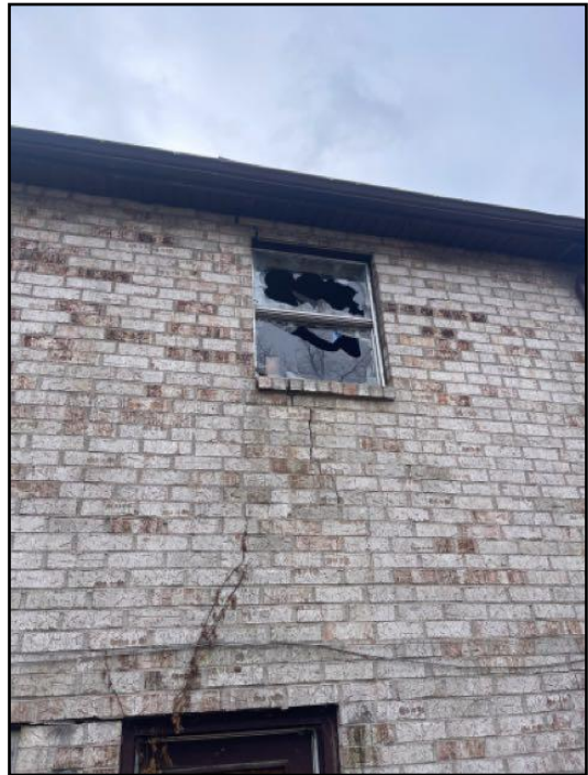
132. The window will cause loss of energy...
