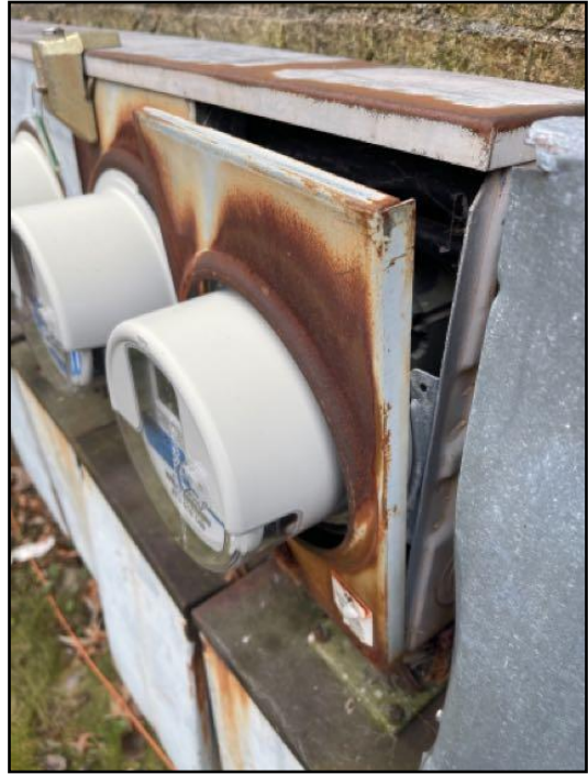
5. Electric panels, meter boxes, junction...
