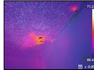
78. Water stains observed on the ceiling could...
