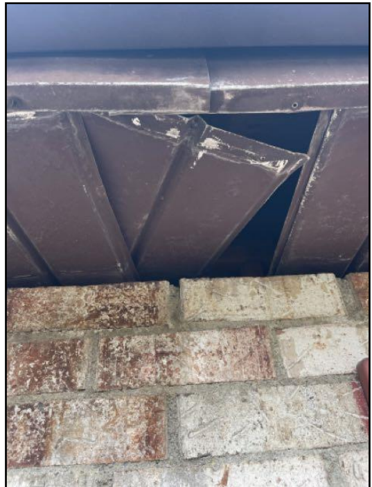
111. Siding has minor damage. Any opening should...
