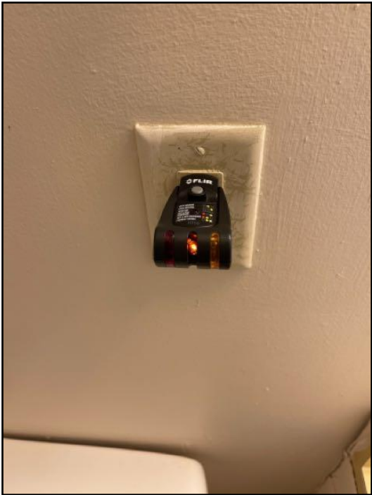
29. .The GFCI is not tripping (shutting off the...
