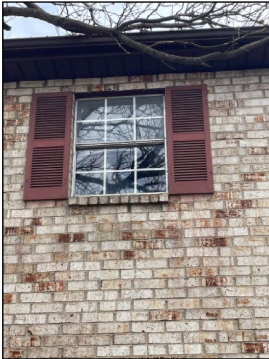
135. The window will cause loss of energy...
