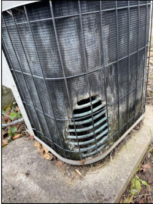
39. Condenser coil damaged / obstructed / dirty
