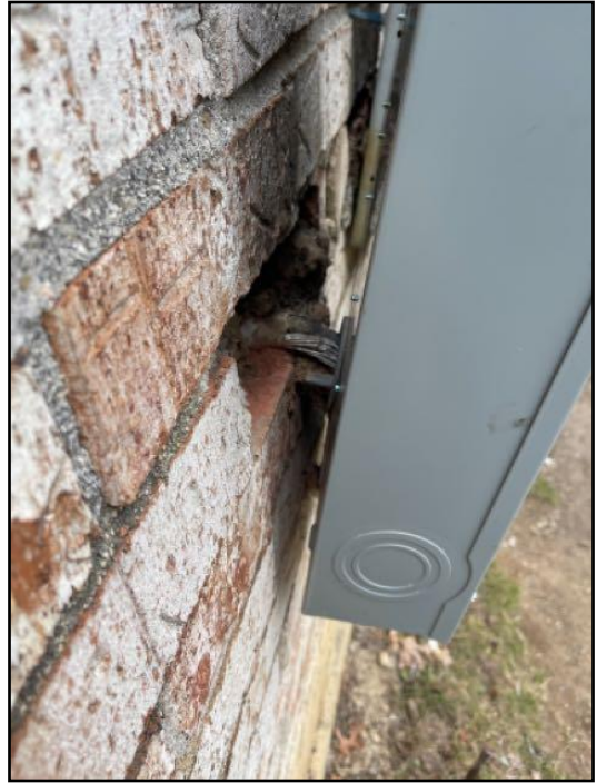
13. Electric panels, meter boxes, junction...
