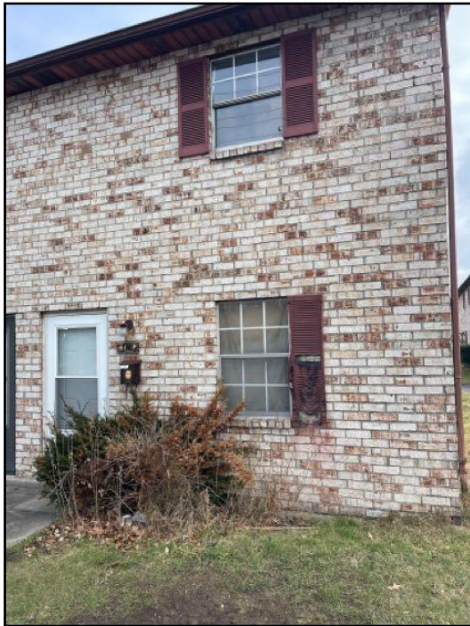
88. Fire damage was found. Consult the owner fo...
