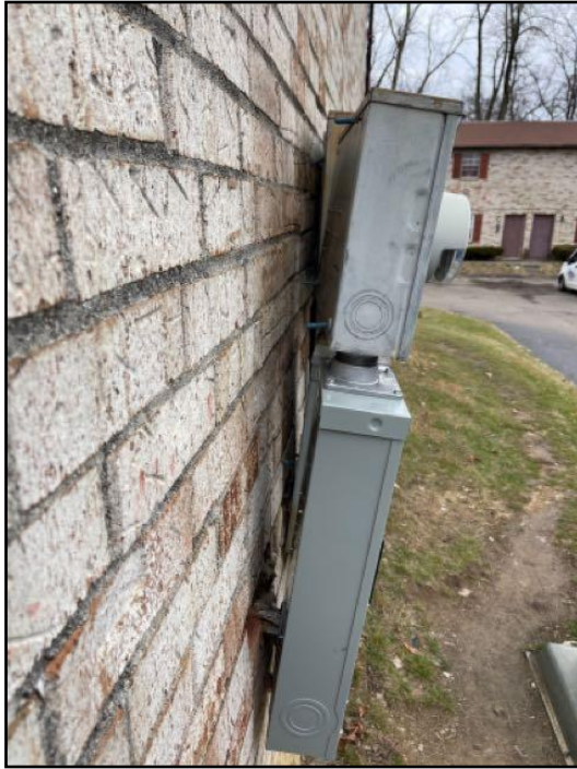
12. Electric panels, meter boxes, junction...
