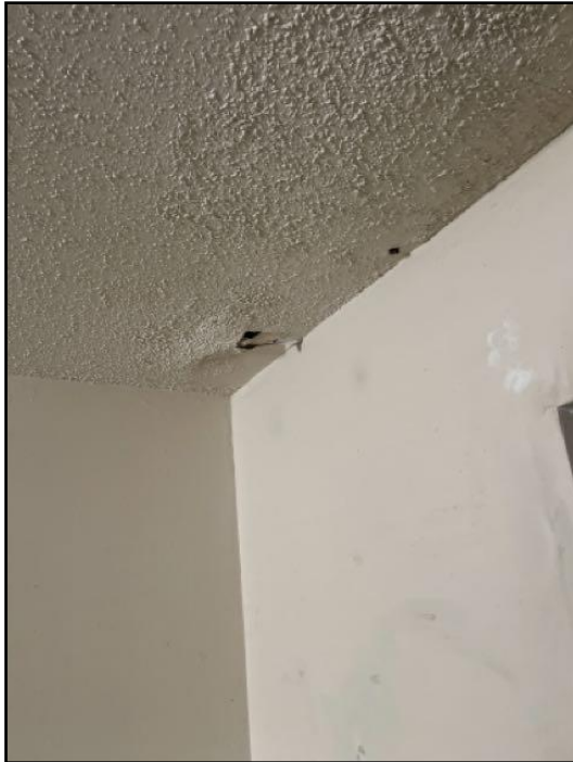
77. Water stains observed on the ceiling could...
