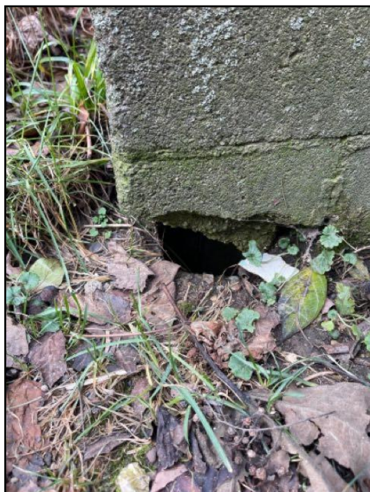
100. Surface deterioration ( spalling, crumbling...
