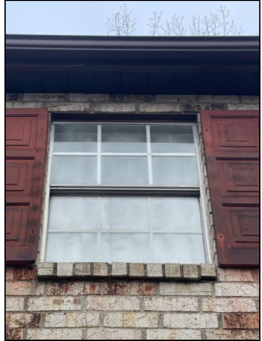
130. Lost seal; formation of condensation between...
