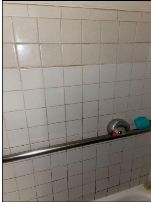
54. Loose tile in the tub/shower enclosure
