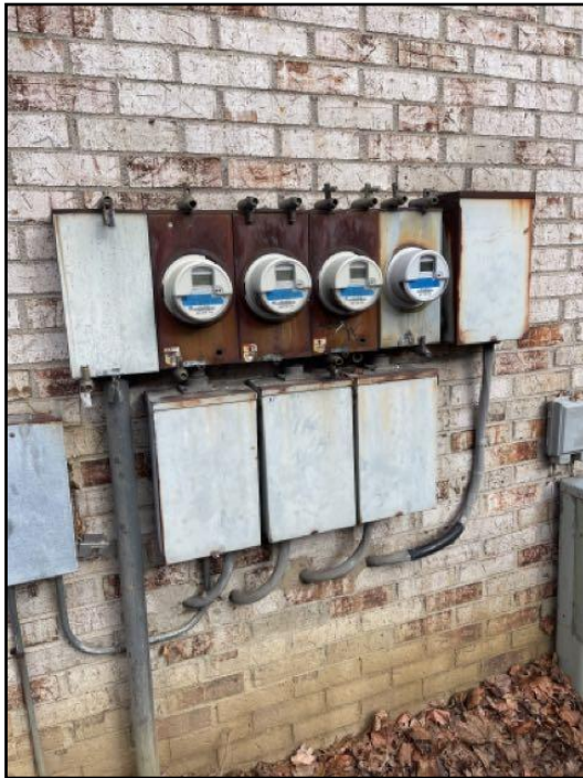
8. Electric panels, meter boxes, junction...
