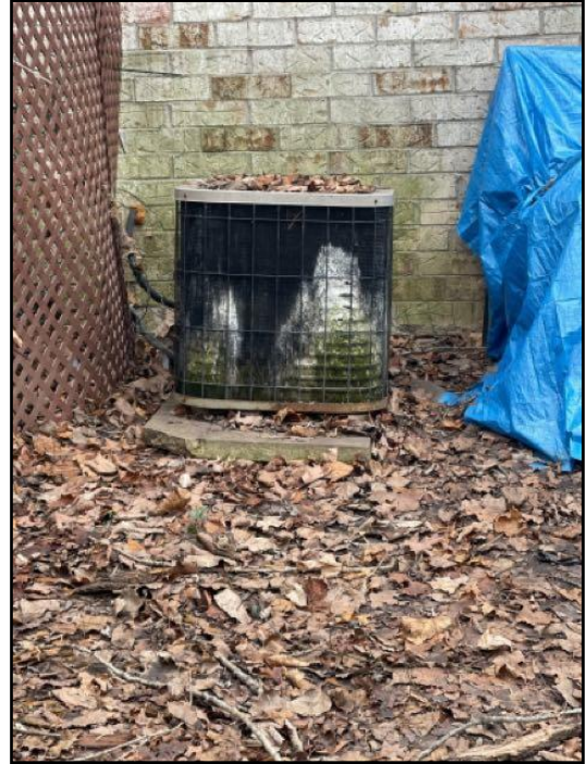
40. Condenser coil damaged / obstructed / dirty
