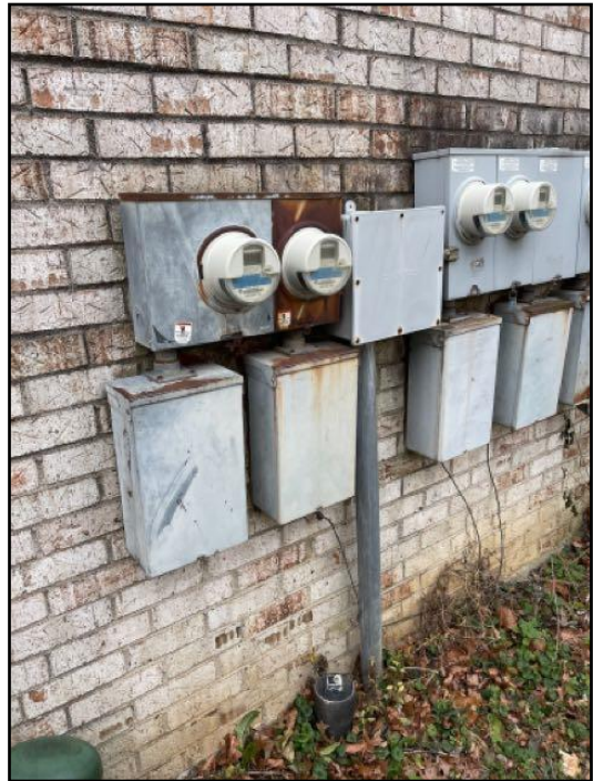
9. Electric panels, meter boxes, junction...
