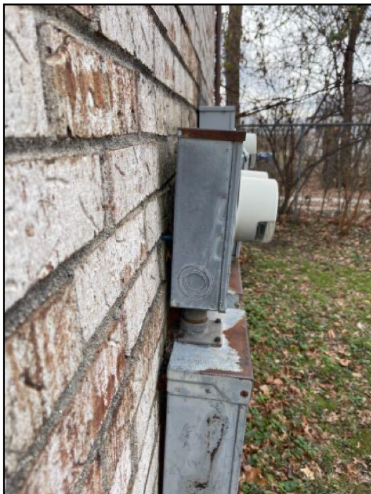
98. Fire damage was found. Consult the owner fo...
