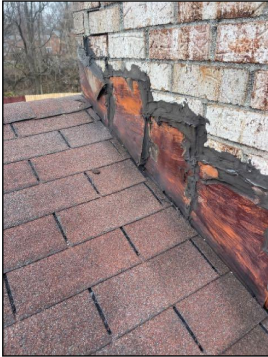
67. Not regletted into the masonry wall
