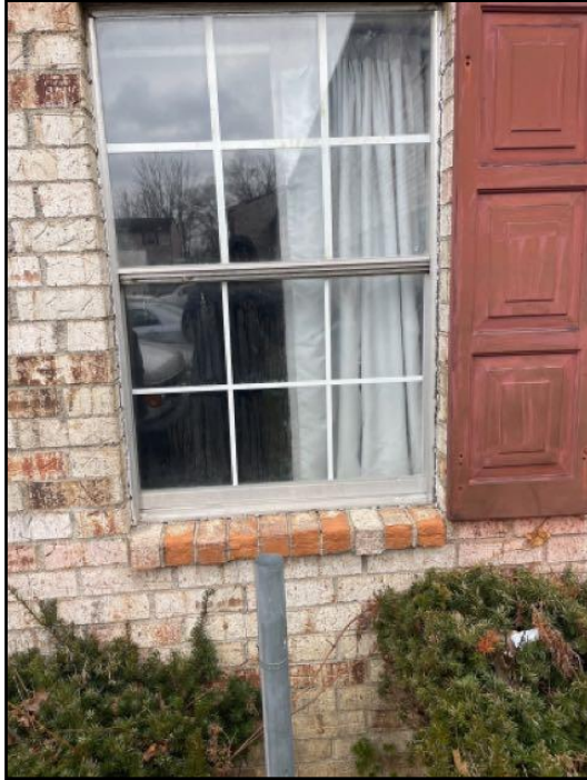
129. Lost seal; formation of condensation between...
