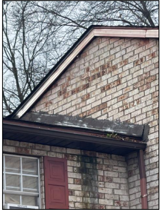
68. Not regletted into the masonry wall
