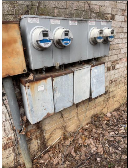
7. Electric panels, meter boxes, junction...
