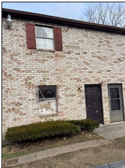
90. Fire damage was found. Consult the owner fo...
