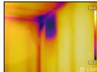
82. Water damage was found at this location...
