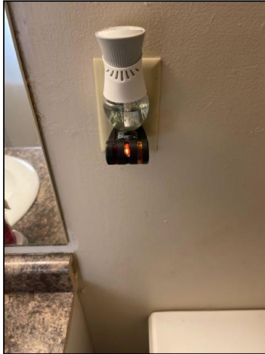
26. Ungrounded three-prong receptacles
