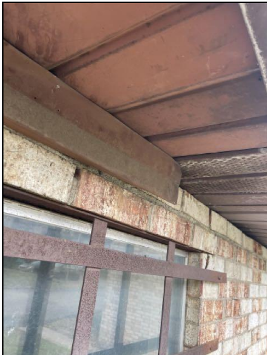
110. Siding has minor damage. Any opening should...
