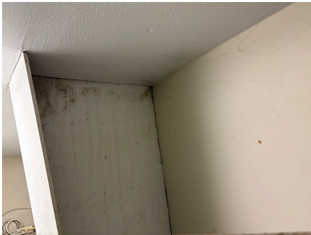
Apparent water intrusion with possible mold growth.
