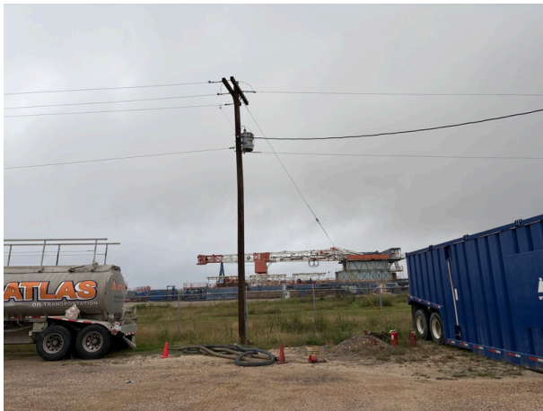
View of pole mounted transformers
