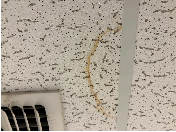
View of stain in the ceiling on the second floor
