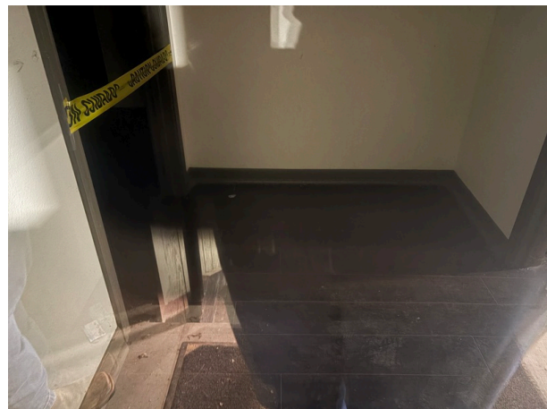
View of closed area due to unstable floor in the second floor in the southern portion of the building
