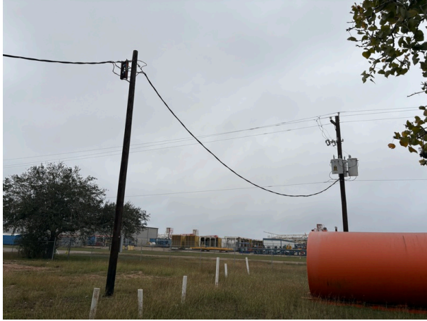
View of transformer
