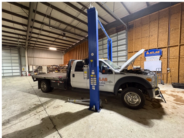
View of lift
