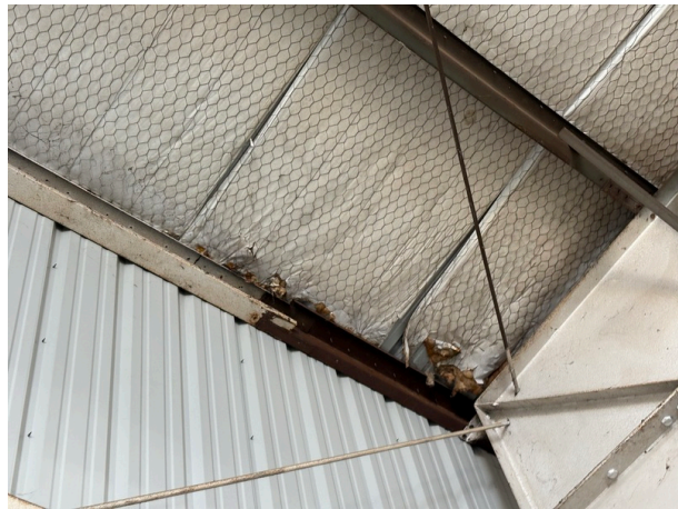
View of stain and crack in the ceiling on the southern portion
