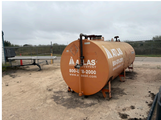
View of 10,000 gallon Diesel AST
