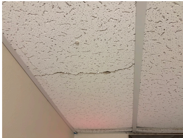
View of cracks in the ceiling on the second floor
