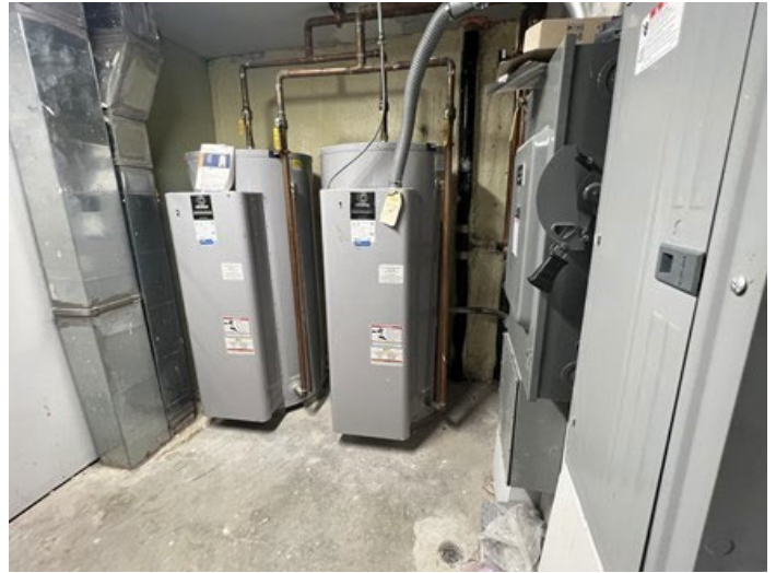
HOT WATER HEATERS
