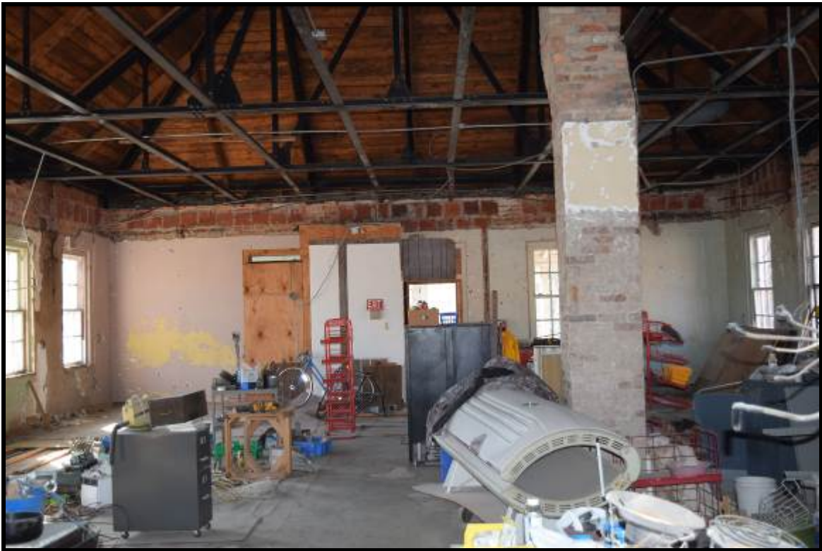
Photo 4: Typical interior conditions in the upper level of the original portion of the hospital.
