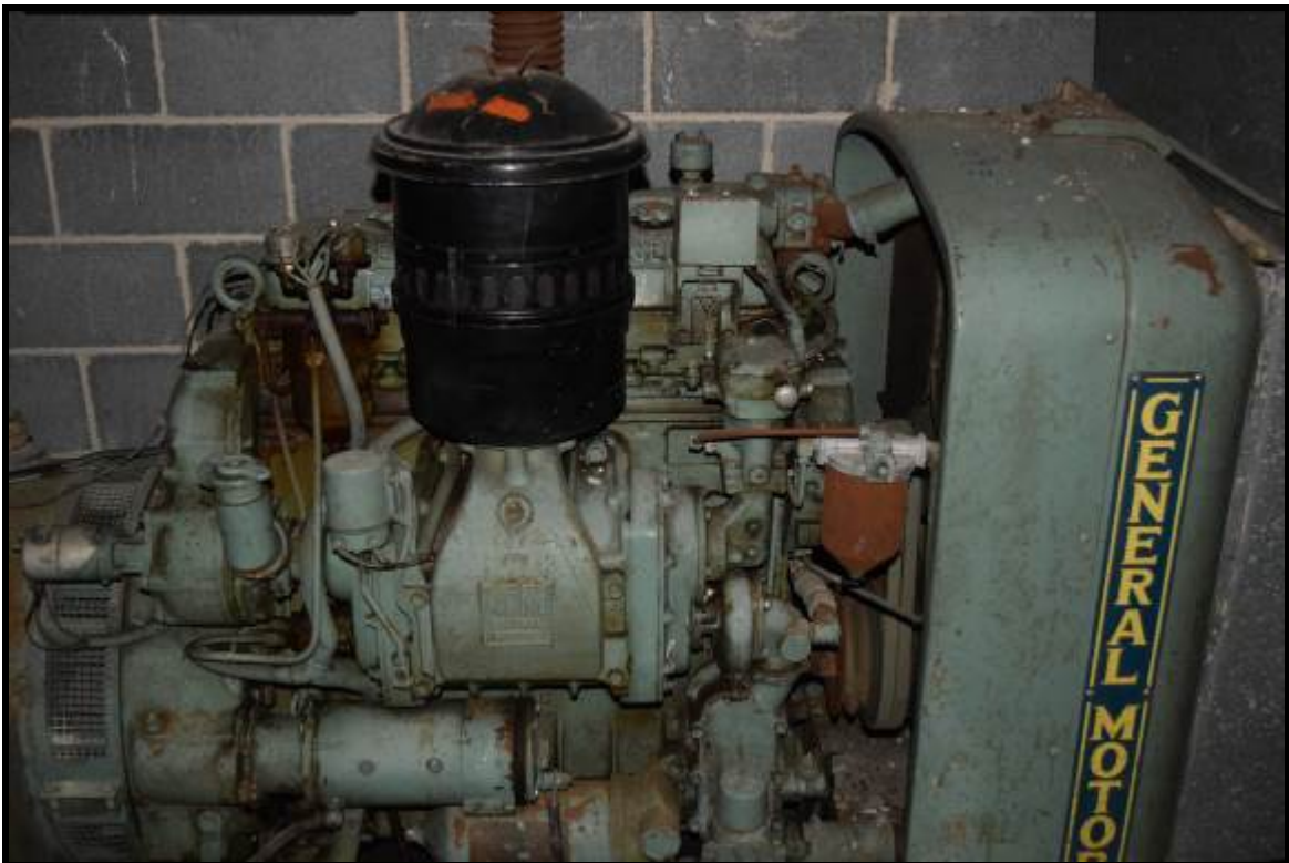
Photo 6: Electrical generator in generator room of lower level of the hospital.
