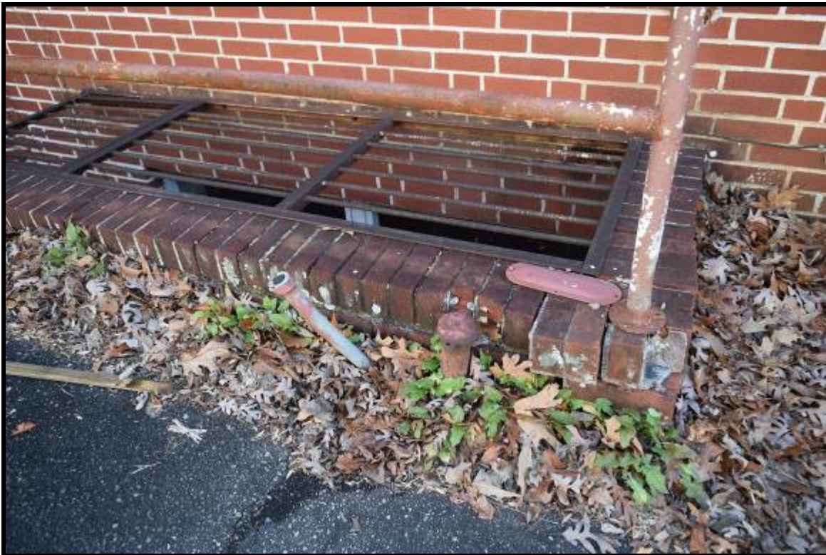
Photo 17: Fuel oil UST vent pipe and fill port adjacent to generator room. Photo is in driveway along west side of south wing addition of the hospital.
