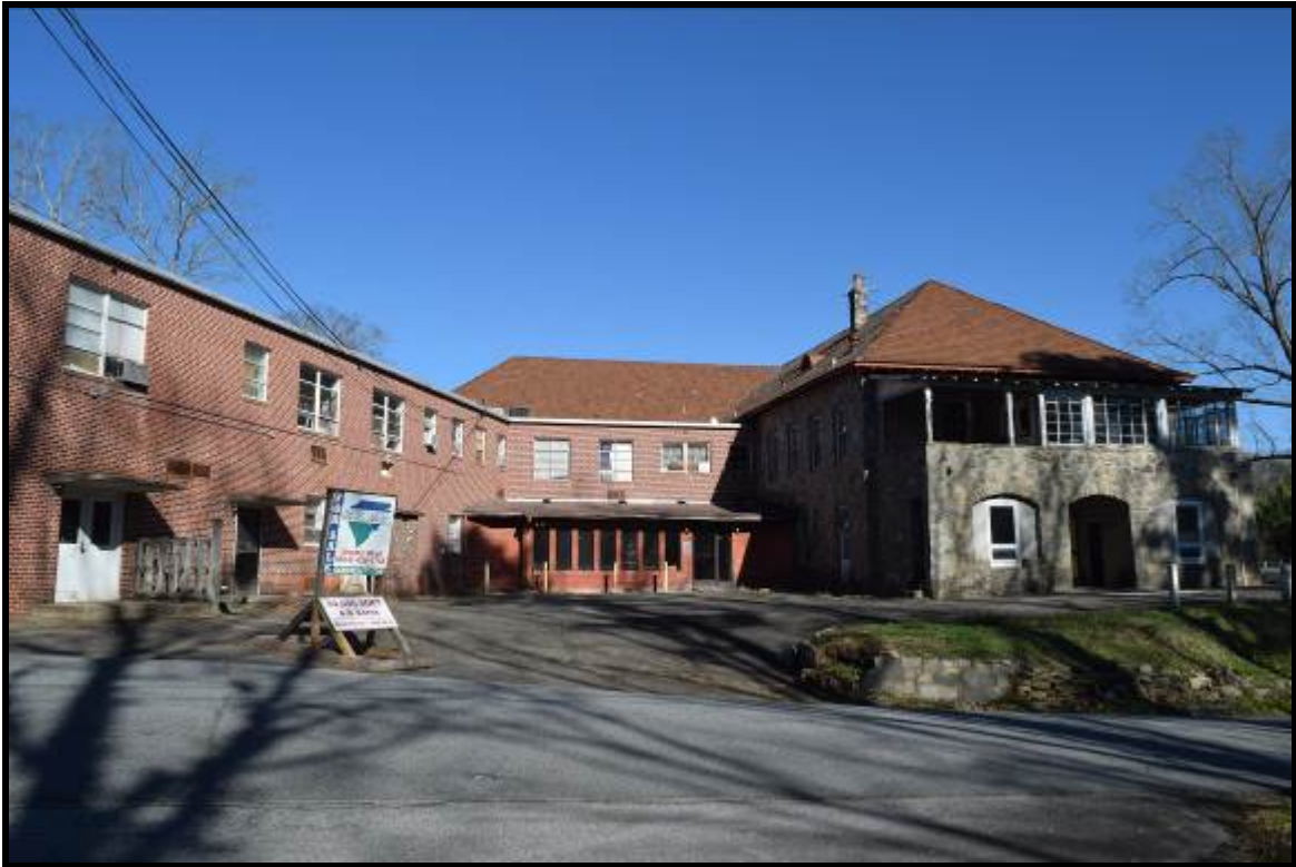
Photo 3: South wing addition to the hospital (central and left portion of photo).
