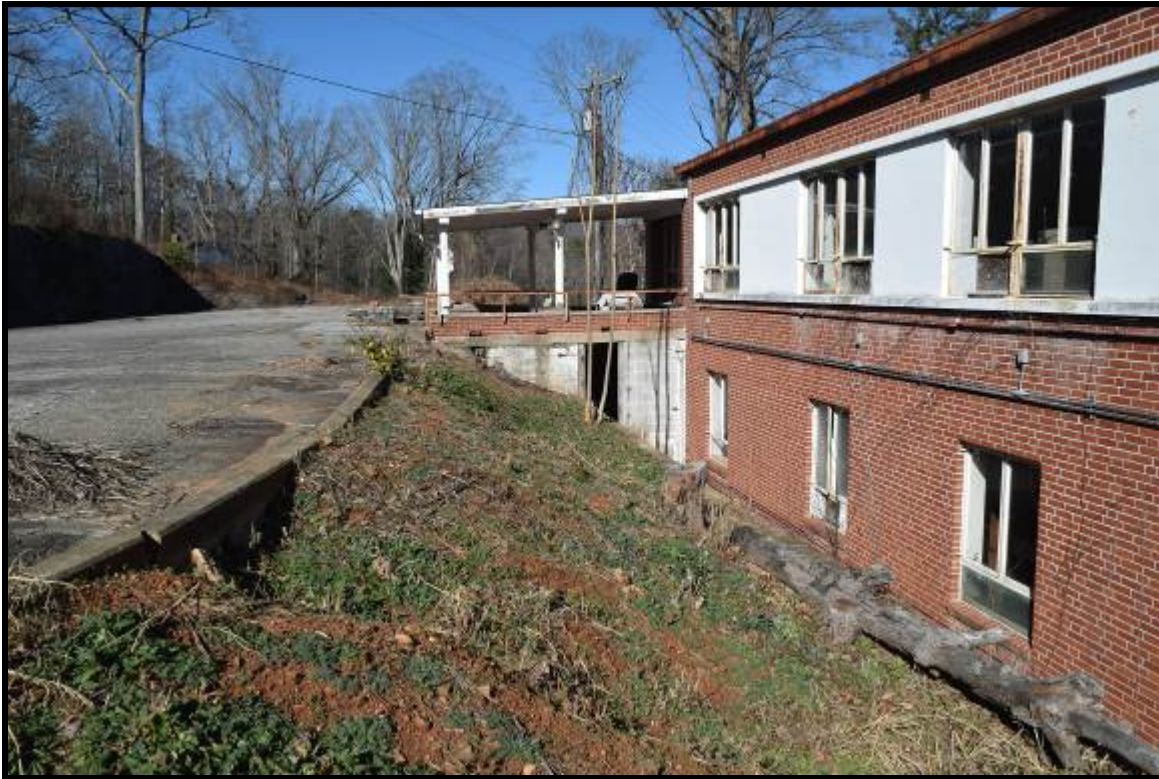
Photo 9: Area of former petroleum (fuel oil) UST vent pipe as seen in 2012 ESA photo. Based on loose soil conditions along the vegetated bank and results of multiple soil borings, it appears the UST in the area was removed between 2012 and the present time.
