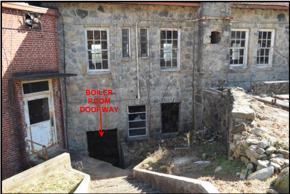
Photo 8: Exterior access to boiler room at north end of west side of the original portion of the hospital.
