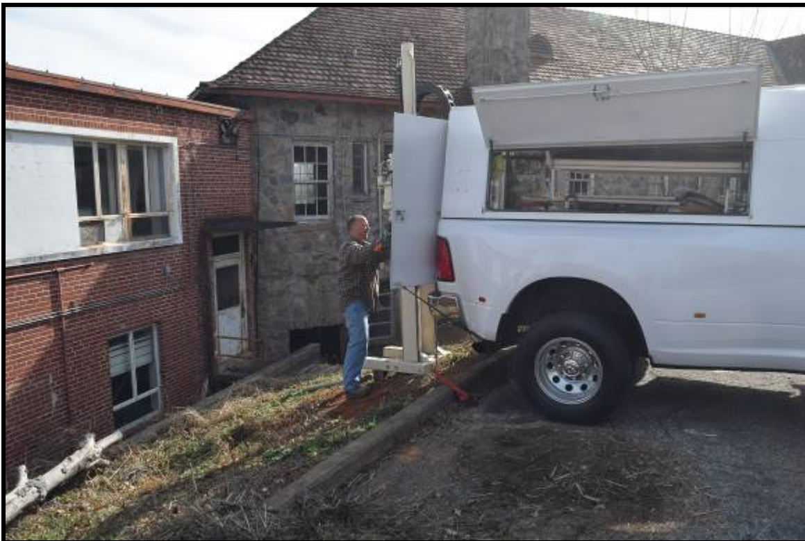
Photo 18: View of driller collecting soil samples in the estimated vicinity of the former fuel oil UST associated with the former boiler.
