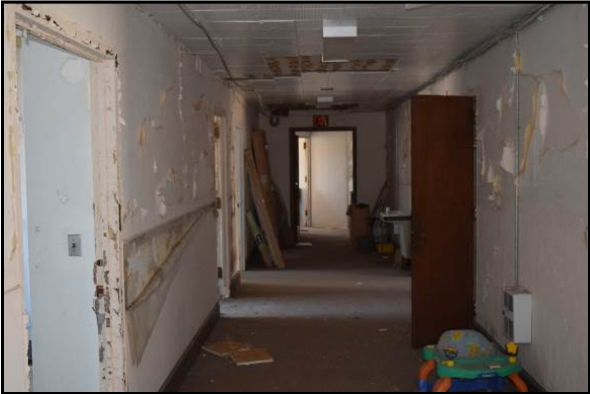
Photo 5: Typical interior conditions of the lower level of the hospital showing interior walls intact.
