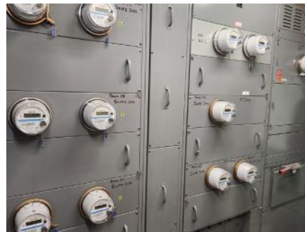
Heavy Power - 3,000 Amps+ Three (3) Electrical Meter Zones Per Floor
