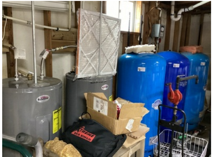
Water Heaters and Pressure Tanks
